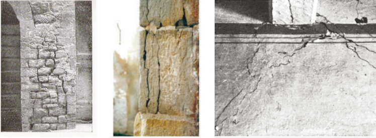
Figure 3. Crushing due to compression.
