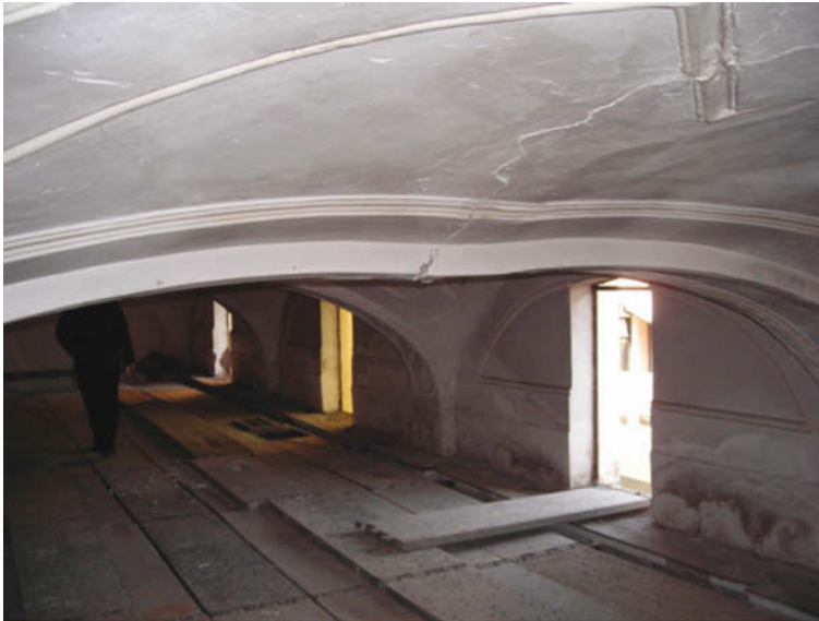
Figure 6. Incipient failure of a shallow cross vault due to excessive spread of the abutments (aisle vaults of a XVI century chapel in Nocera Inferiore (SA), Italy). Courtesy of Enrico Sicignano.
