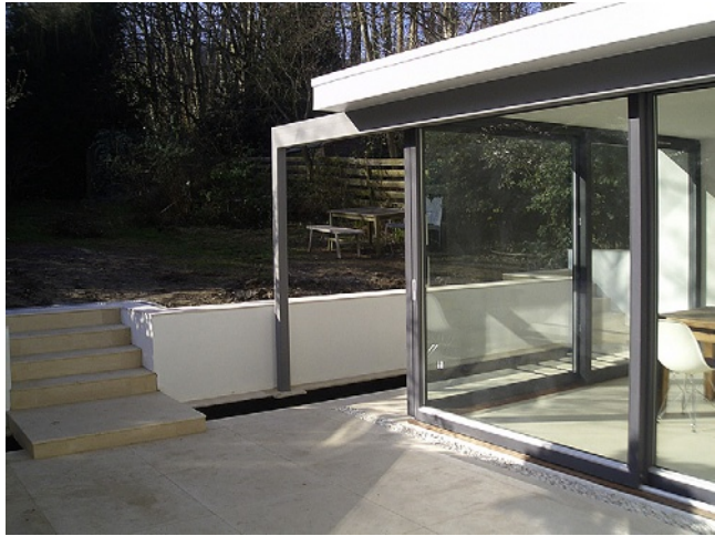
Figure 3.2 Extension: Bowkett, Tankard Architects. This simple and elegant back extension has been structured using steel beams and posts. The main support has been taken outside the building envelope and has been made a feature so that the roof looks as though it is floating, and enables the corner of the building to be opened up to dramatic effect. © Bowkett, Tankard Architects
