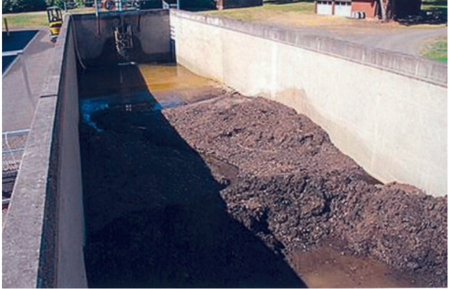
FIGURE 12-16 Settling ponds allow solid material to settle to the bottom. Eventually, they have to be cleaned.
