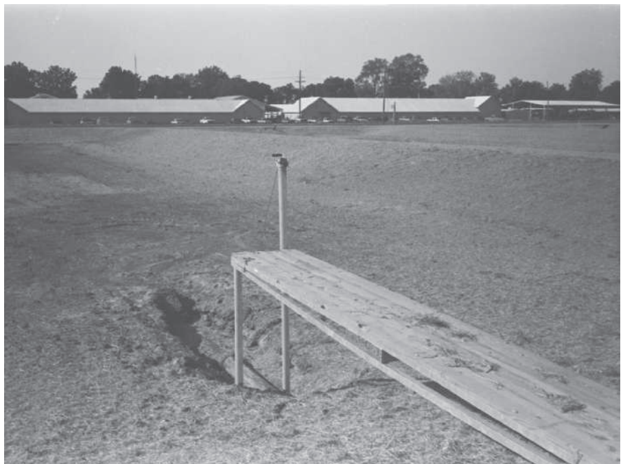
FIGURE 13-11 Swivel drain in a newly constructed pond. Pipe is lowered to drain the pond.
