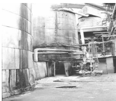
Figure 23.1. Leakages at a production plant
