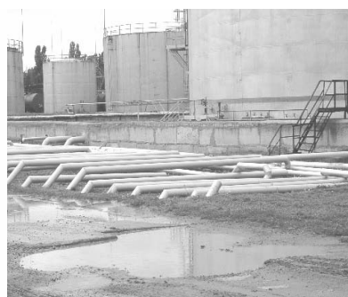
Figure 23.2. Single wall pipe subways through retention room; no knock-down protection
