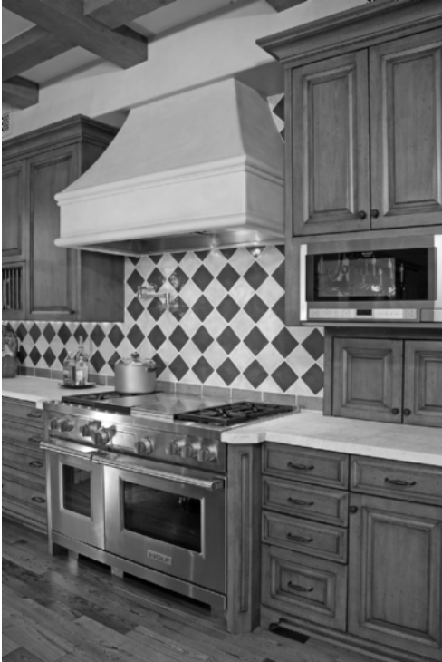
Figure 5-20 A range installation. (Photo courtesy of Mary Fisher Designs. com, Northlight Architectural Photography. com)
