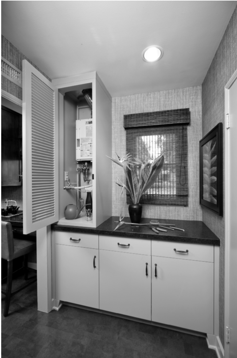
Figure 12-1 Tankless water heater installed in place of the standard tank water heater, allowing additional space for storage and counter. Louvered door provides air circulation. (Photo courtesy of Judy Svensen, Raven Interiors, Mary Fisher Designs.com, Gary Milici Photography)
