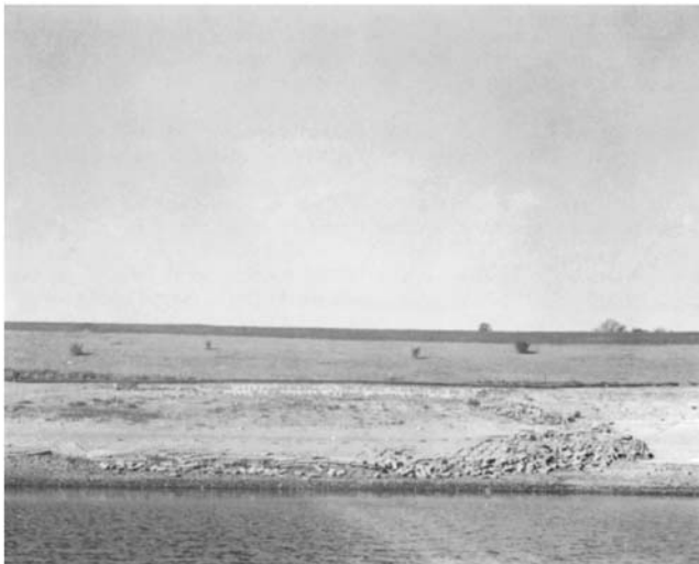
Figure 8.11 Slumping of the interior lining of a reservoir. Part of a photograph taken with a UMK 10/1318 camera from a small dinghy.
