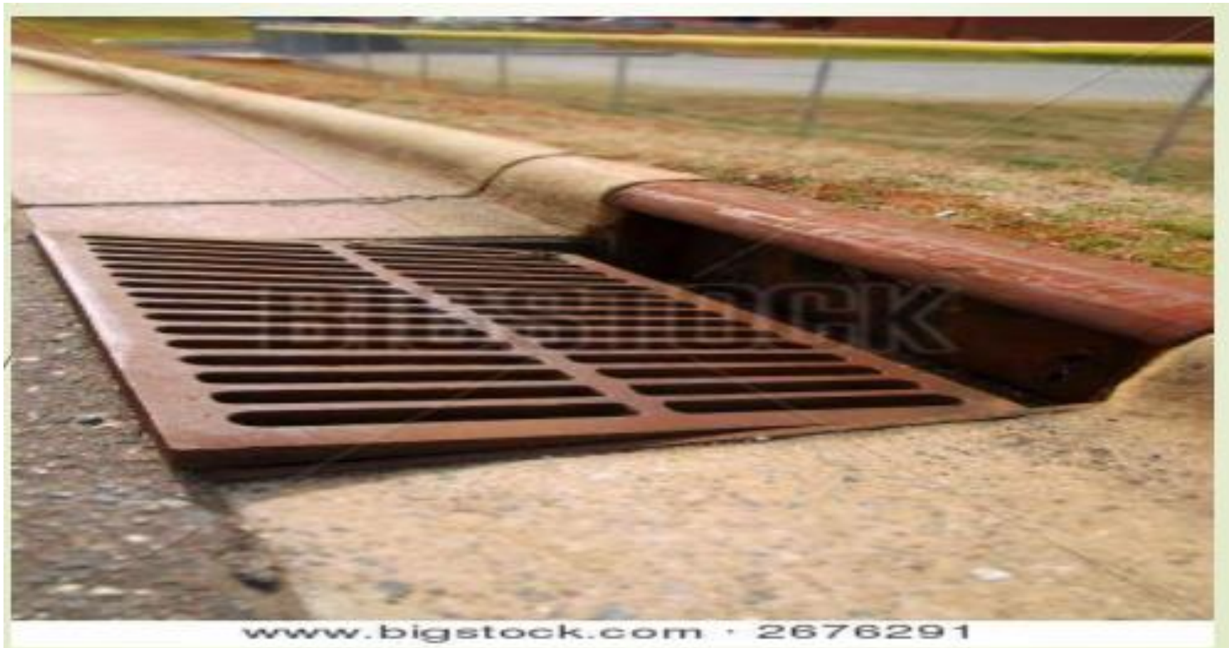
Fig 2.3 b) Showing road side gutter of storm water collection system
