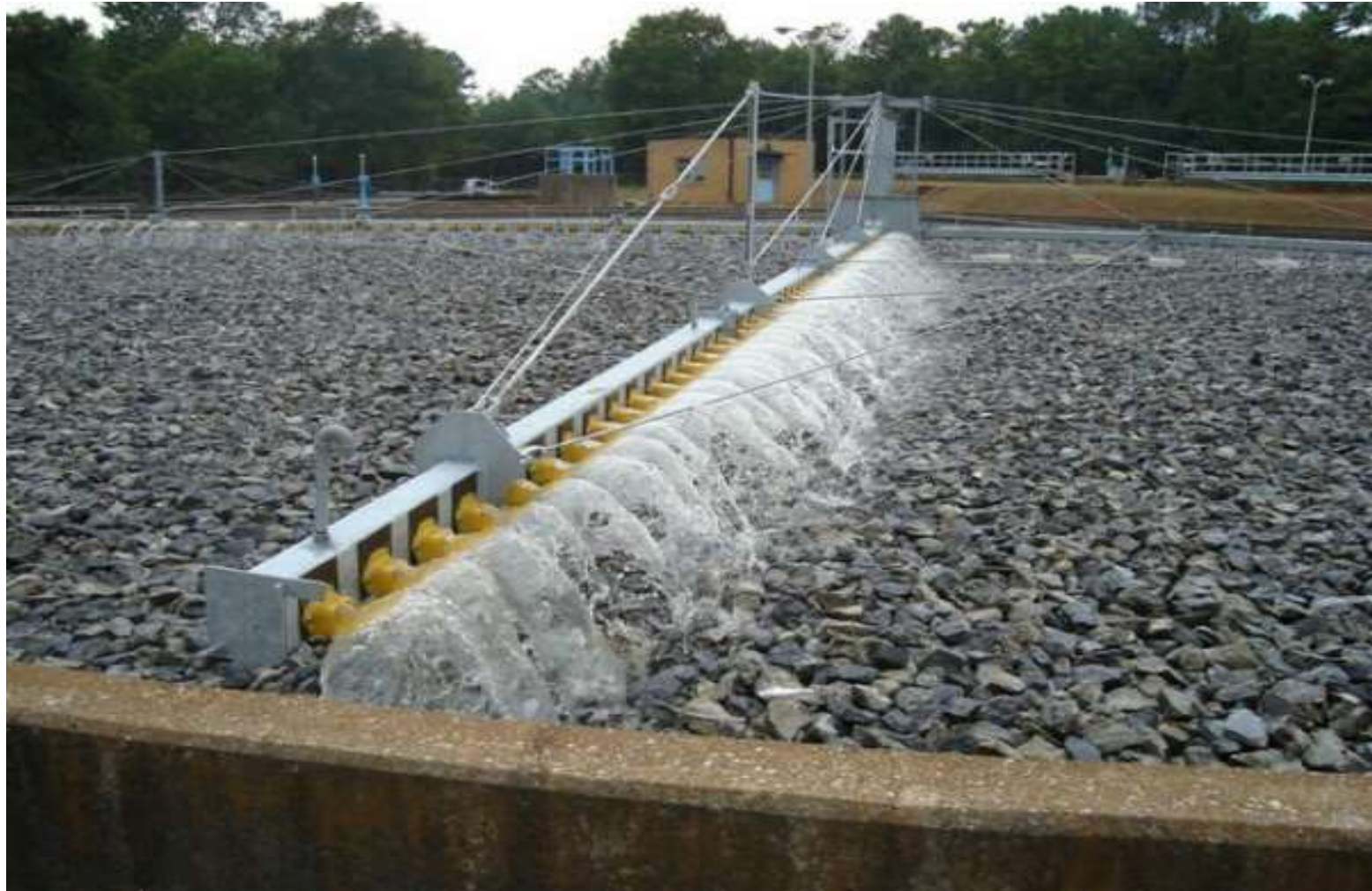
Figure of Photographic view of trickling filter with its rotary distributors
