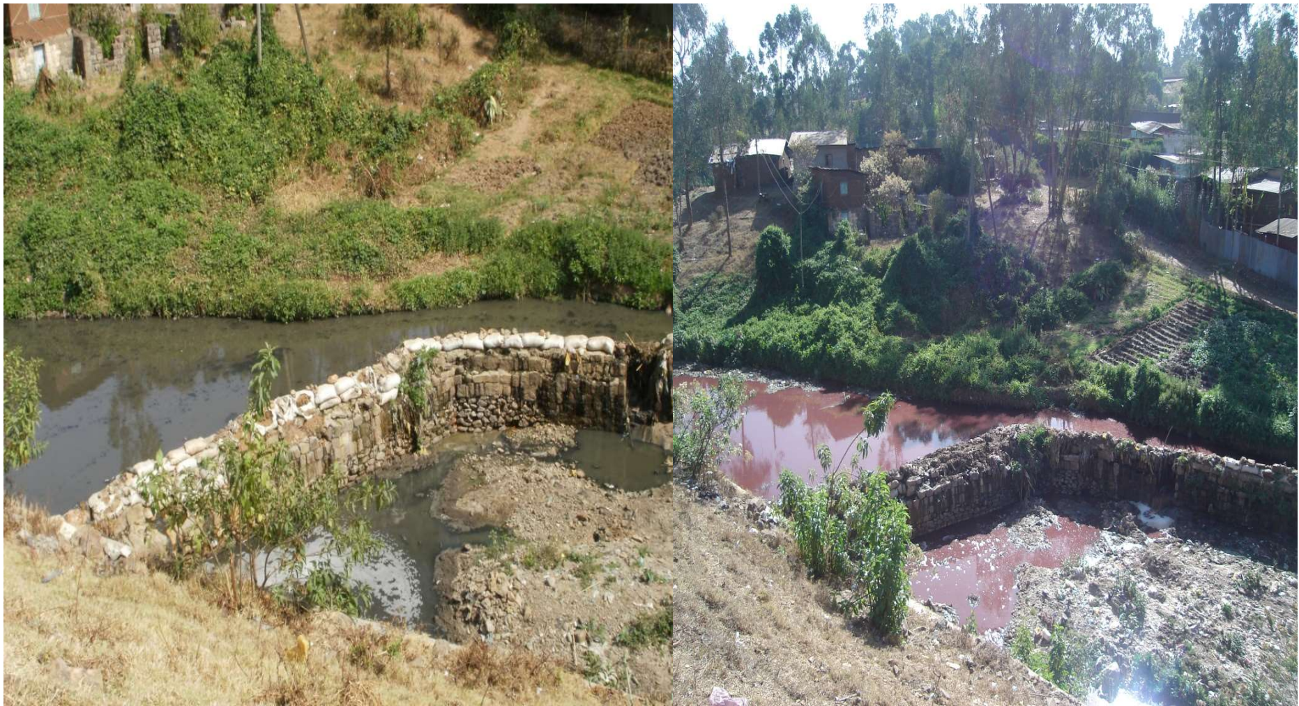
Photo of Kaliti (A.A)WSP- effluent diversion weir for irrigation
