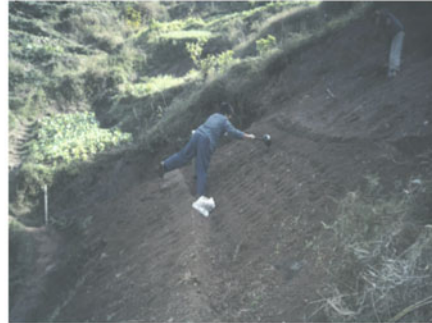
Reclamation of sloping land with a gradient bigger than 40 degrees at Tangpu village in the town of Changling
