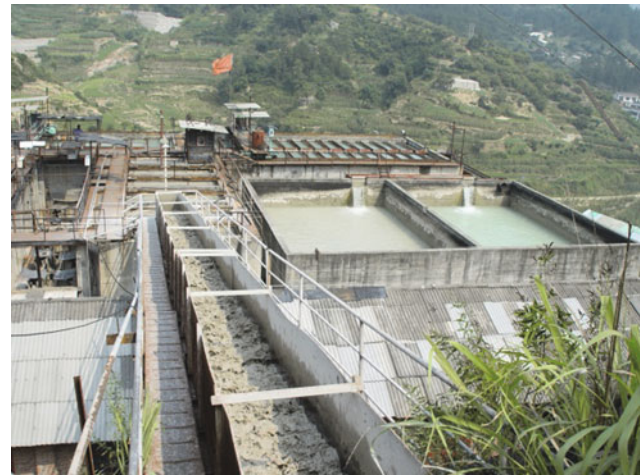
Waste water treatment of sand washing and reclaimed water recycling pools
