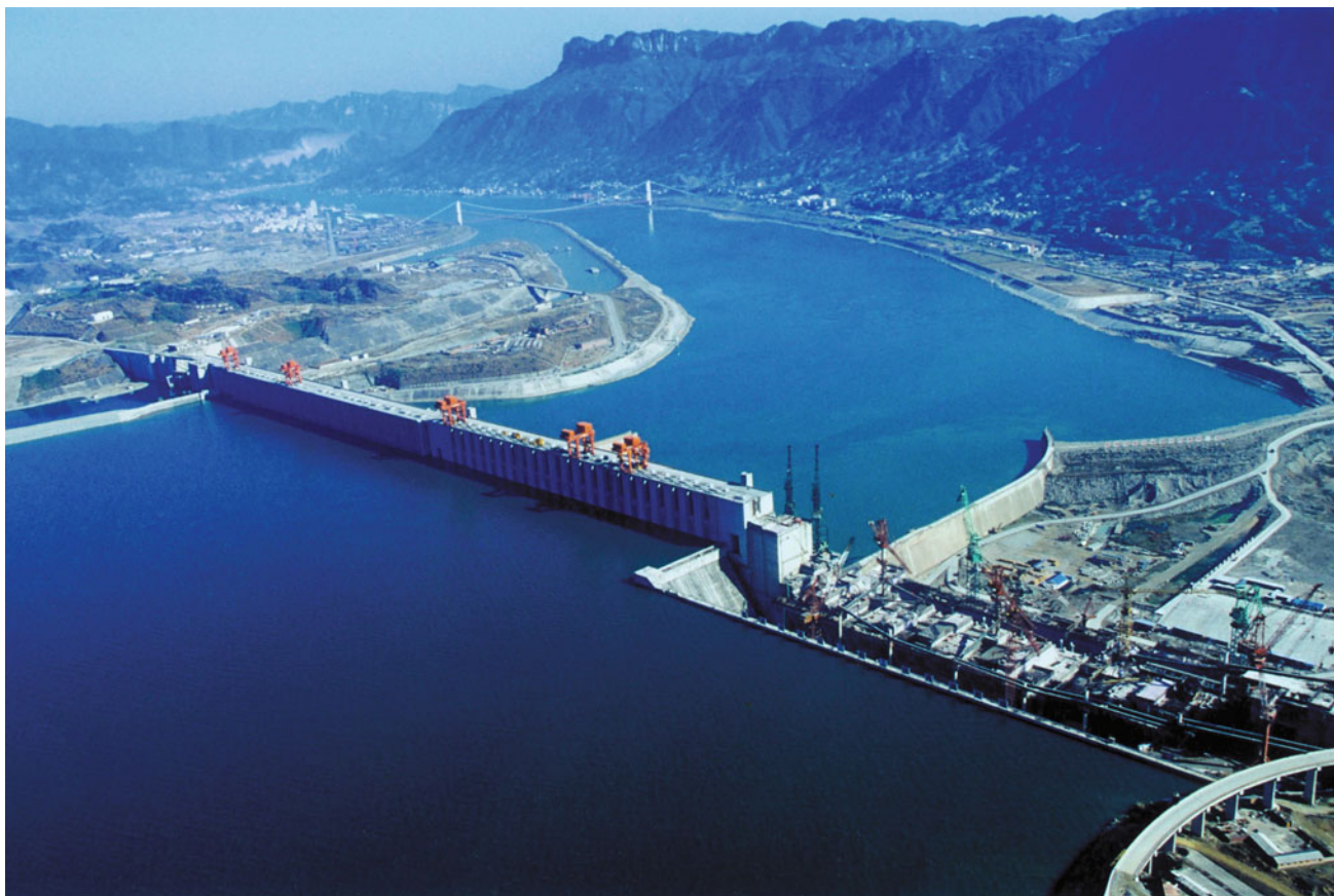
Three Gorges Dam holding water. The barrage structure on the left bank is completed and those on the right bank are still under construction. (Photo by Xinhua Reporter, May 2005)
