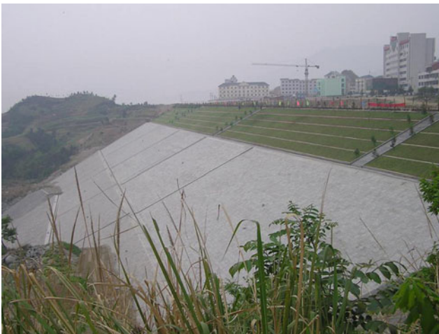
Project for protecting the reservoir bank at the Town of Taipingxi, Yiling District of Yichang City
