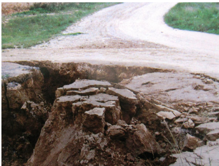
Fig. 1.19 Loess collapse caused by road scouring. From Zhu (1986)
