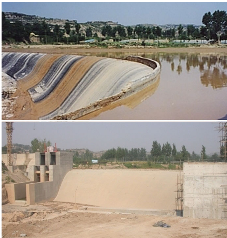
Fig. 7.4 Luohui irrigation district water withdrawal facilities (upper, before improvement; lower, during improvement. Completed in 2006)
