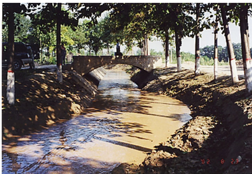
Fig. 7.6 Luohui irrigation district, Ludong block central main channel (lining is damaged in this section)
