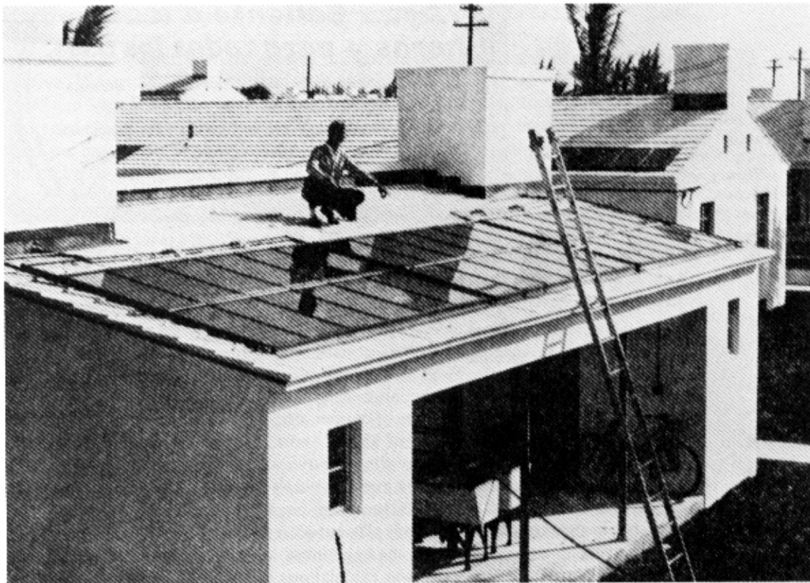
Below: Workman installing solar water heaters in the roof of the laundry room in a Florida subdivision built during the late 1930's. Every home in this tract had its own solar water heater.
