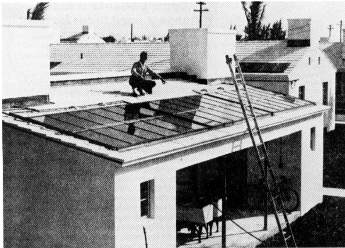
Below: Workman installing solar water heaters in the roof of the laundry room in a Florida subdivision built during the late 1930's. Every home in this tract had its own solar water heater.
