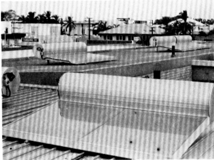
This group of solar heaters provided hot water for the Don Hotel in Darwin, Australia.
