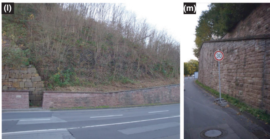
Fig. 6.1 Case history of landslide impacts for the landslide site “Altmündener Wand” at the highway B 3 in Hann. Münden, Upper Weser area (Photos Database B. Damm; M. Grochau, photo: g)
