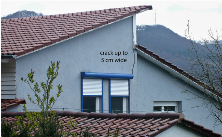
Fig. 3.9 Crack in a house due to slope movements
