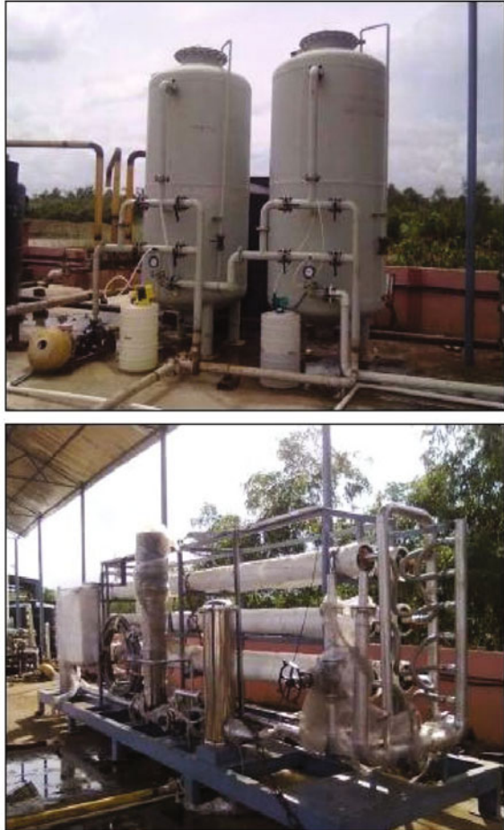
Fig. 10 Facility for reverse osmosis (RO) of CBM-produced water at Raniganj (Courtesy Drinking water project-Essar Oil)
