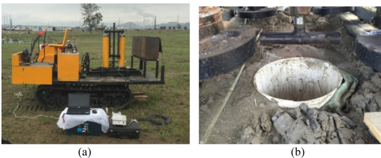
Fig. 5. (a) Equipments, (b) Pre-embedded pipe
