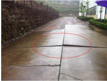
Fig. 3. Arching of concrete pavement
