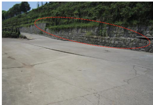
Fig. 6. The deflection of retaining wall
