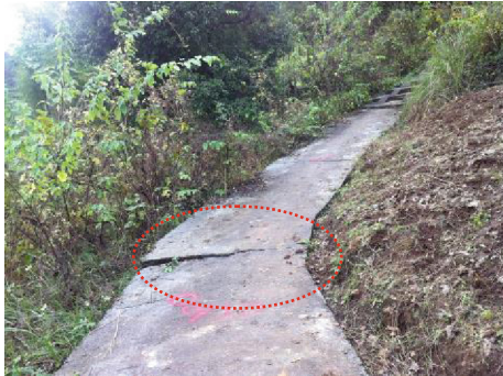
Fig. 4. Cracking of concrete pavement
