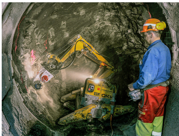
Fig. 2 Photo (by COMET) of the excavator (equipped with a small rotary drum cutter) used in the FE tunnel mainly for profiling
