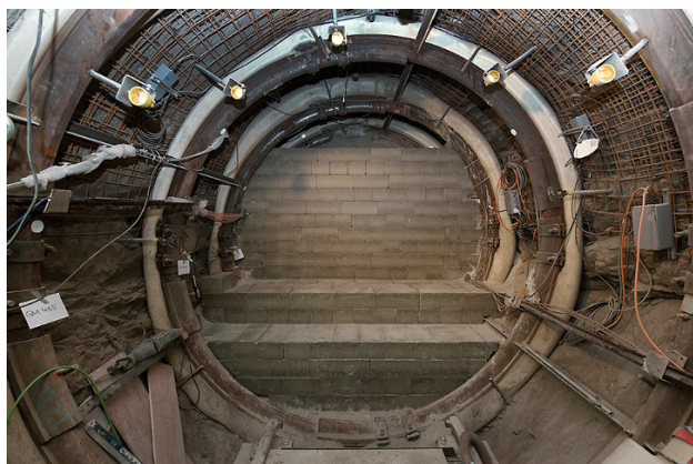
Fig. 17 Photo (by COMET) of the unfinished bentonite block wall in the 'interjacent sealing section' (ISS) at the deep end of the FE tunnel
