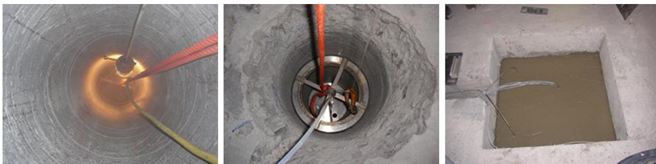
Fig. 17 View into borehole SB2 (diameter 300 mm) after emplacement of sand/bentonite mixture ( left ), after installation of the packer ( centre ), and after grouting of the borehole cellar ( right ) (Rothfuchs et al. 2012)
