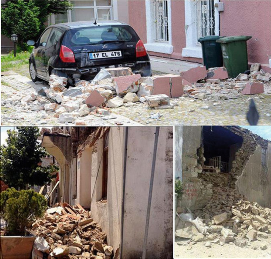
Fig. 17 Some examples of heavily damaged house from Gökçeada Island and Çanakkale (Turkey; by AA)
