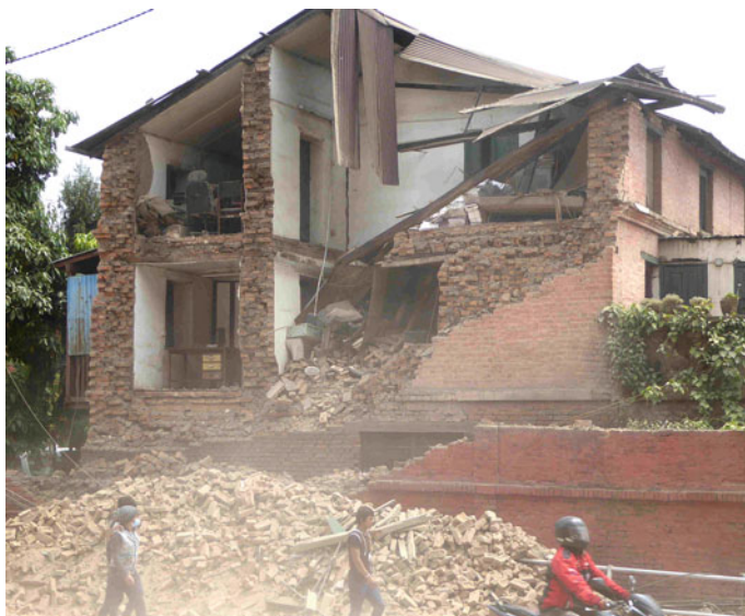
Fig. 2 Collapsed front section of a house built completely of bricks without further enforcement; Jamal, Kathmandu, Nepal. Photo JH Kruhl (26 April 2015)
