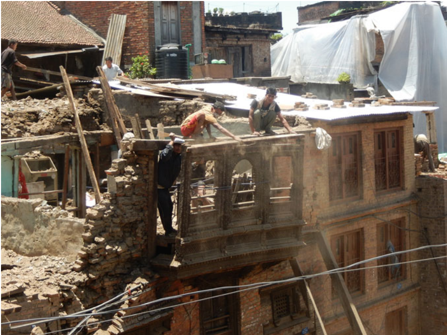
Fig. 3 Volunteers, students and workers taking extra care to remove the window frames
