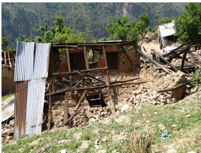
Fig. 3 Collapsed house built of stone masonry; village east of Melamchi, Melamchi valley, northeast of Kathmandu, Nepal. Photo JH Kruhl (1 May 2015)
