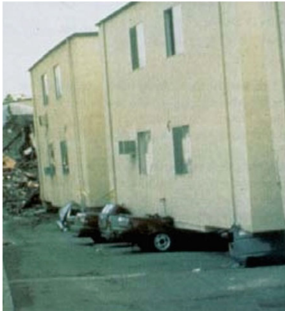
Fig. 2 Soft storeys are an important architectural requirement. They are one of the most dangerous features but there are no design rules for them in codes: Instead, they are forbidden (from EERI slide collection)
