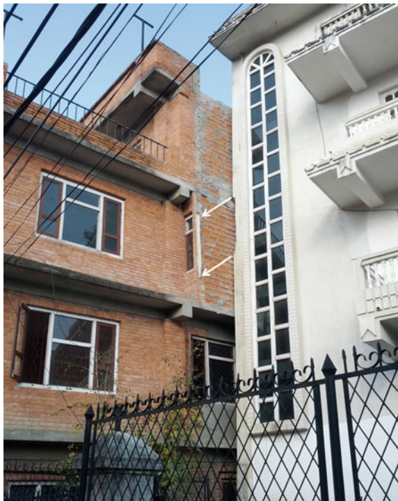
Fig. 1 Tilting and subsidence caused by the Gorkha 2015 earthquake; four-story building in Lokanthali, south of Tribhuvan Airport, Kathmandu, Nepal. The white arrows indicate the tilting and subsidence path of the left building. Photo JH Kruhl (2 May 2015)
