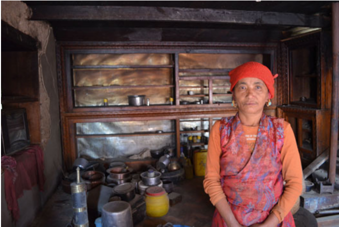
Fig. 1 A woman stands inside what used to be the kitchen in her badly damaged and uninhabitable home
