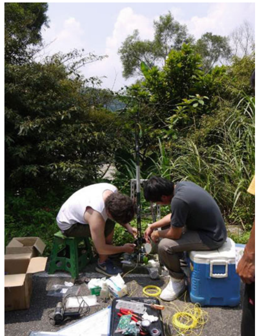
Fig. 22 Field installation of an FBG in-place inclinometer on the Hua-Fan university slope
