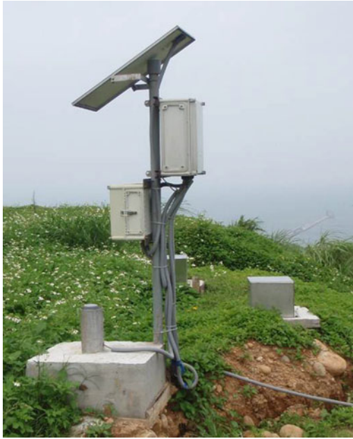
Fig. 9 A fully automated field monitoring system
