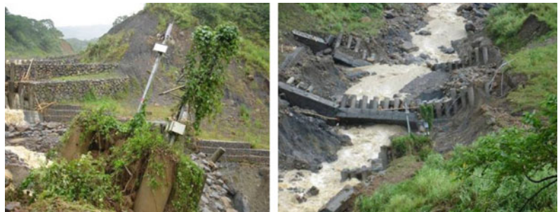
Fig. 22 Damaged equipment and site condition after Typhoon Kalmaegi
