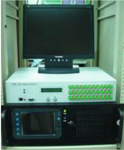
Fig. 14 The fibre optic Bragg grating (FBG) data logging system
