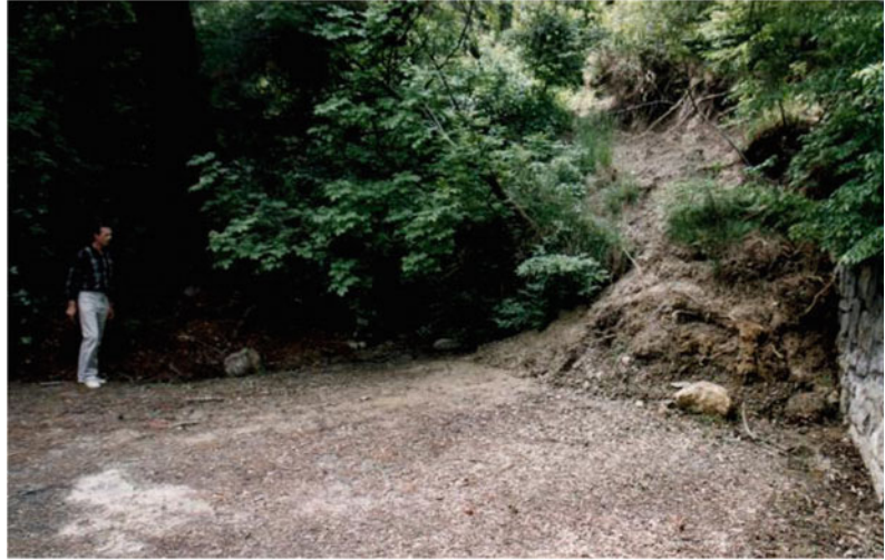
Fig. 7 Cutting of the road with external retaining walls by the “West” landslide left border
