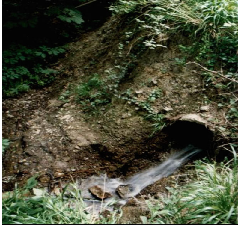
Fig. 9 Broken down catchwater pipe of the drainage gallery south branch
