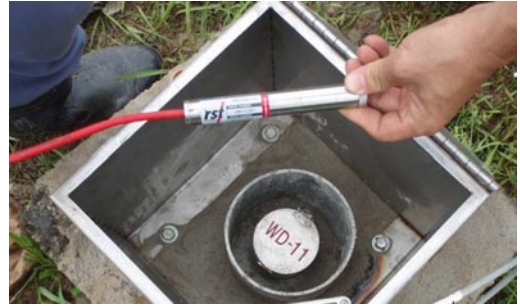
Fig. 11 The vibrating wire piezometer (DECL, Taipei, Taiwan)
