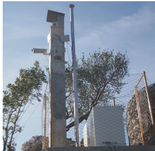
Fig. 5 The master unit consisted of the robotic total station, single frequency GPS master unit, meteorological sensor, and web cam
