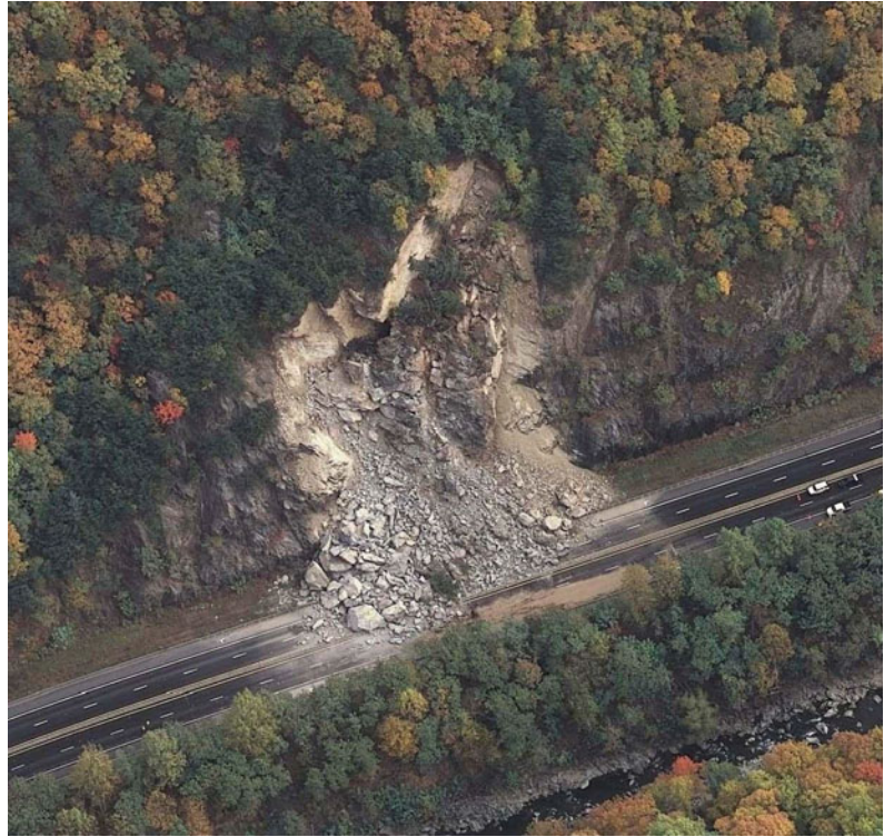
Fig. 3 This rockfall in North Carolina (USA), occurred on a highway through Pigeon River Gorge, on October, 2009, and caused traffic delays for weeks. Photo by North Carolina Department of Transportation
