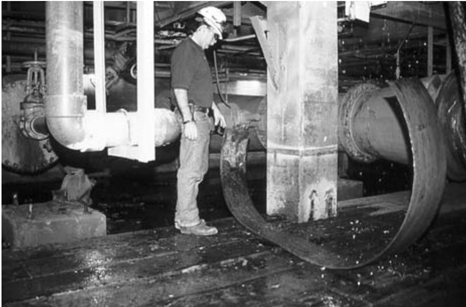
FIGURE 7-10 Photo of how the pump pipe coupling yielded during the explosion.
