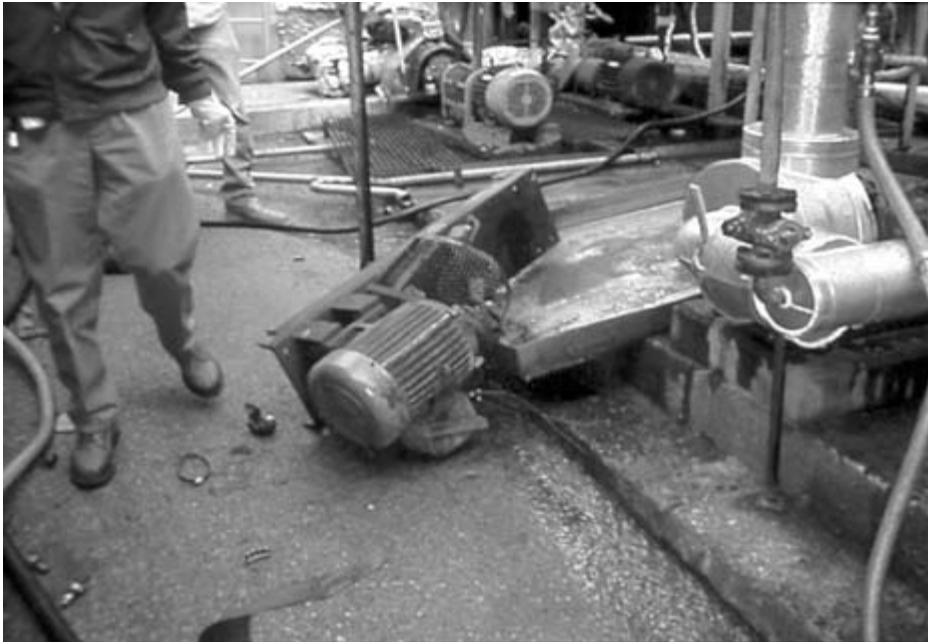
FIGURE 7-13 Pump base plate and motor thrust into walkway. Courtesy of Eastman Chemical Company.
