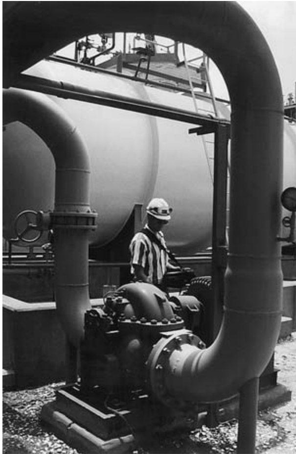
FIGURE 10-2 A vibration technician taking readings on a cooling water pump.
