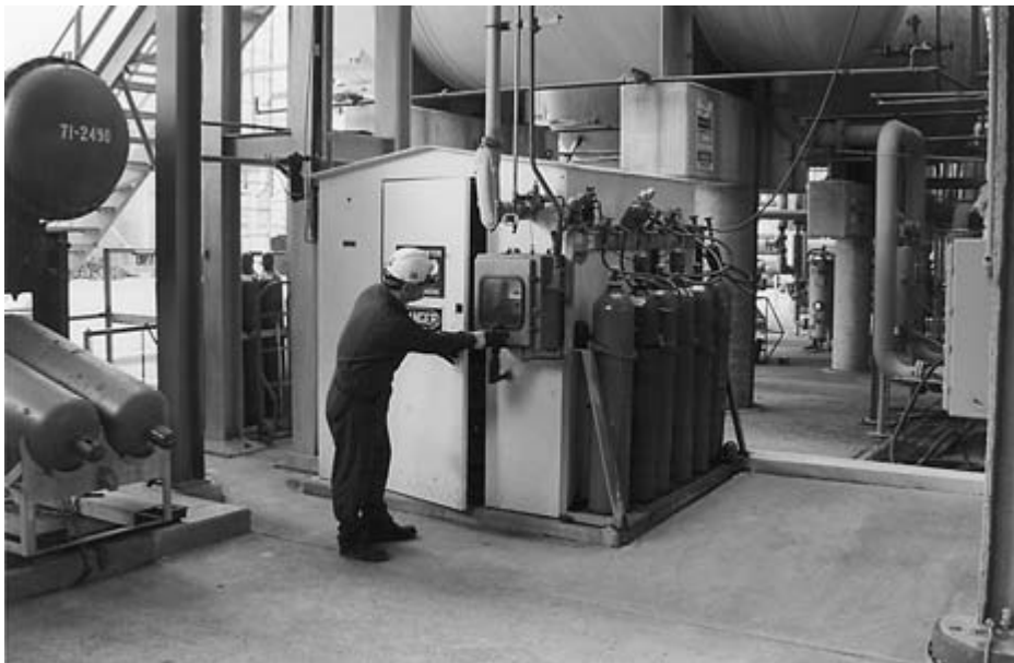
FIGURE 2–23 Typical pressurized and purged analyzer buildings found in chemical plants handling flammables.
