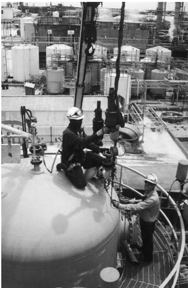
FIGURE 10–20 A mechanic is reinstalling an SRV after it was tested in the shop and raised into position by a crane.
