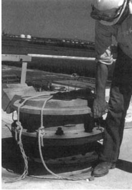
FIGURE 6–10 Hinged vent lid improperly tied to cope with anticipated high winds and to prevent intrusion of rain.
