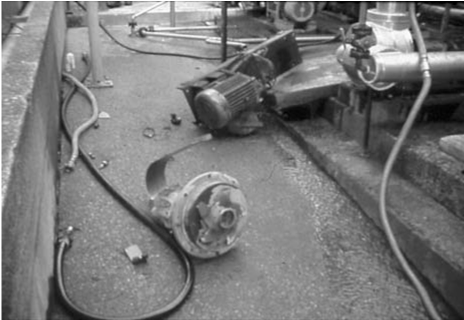
FIGURE 7-14 Pump base plate and motor as well as the position of the bearing housing with impeller document the explosion. Courtesy of Eastman Chemical Company.
