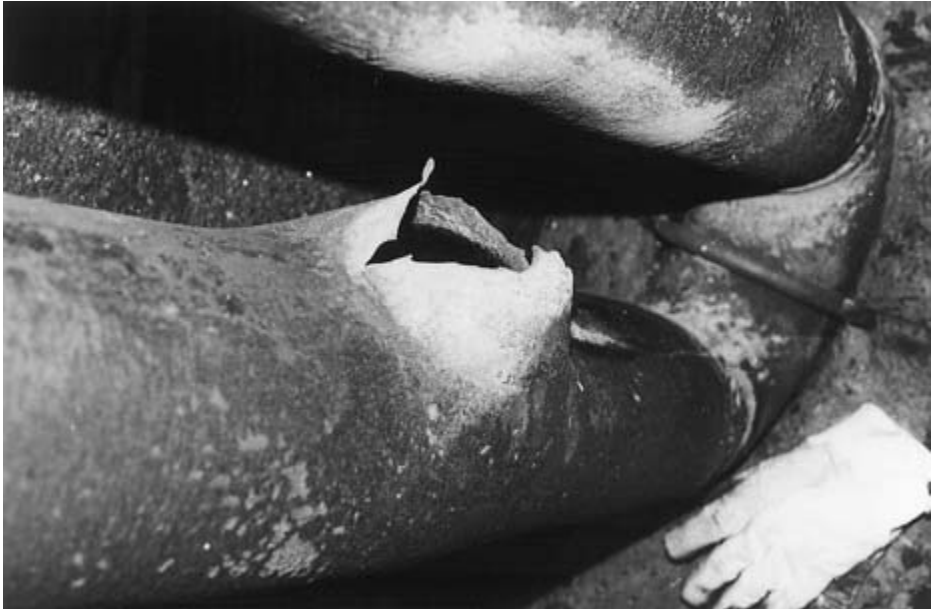
FIGURE 6-2 Tube rupture in a fired heater.
