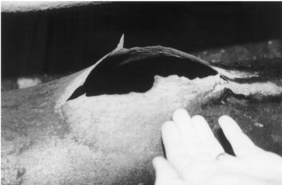
FIGURE 6-3 Close-up of the tube failure.
