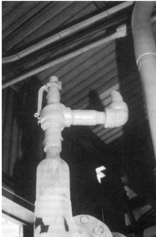
FIGURE 6-13 A threaded safety relief valve reinstalled with a reduced discharge piping arrangement.
