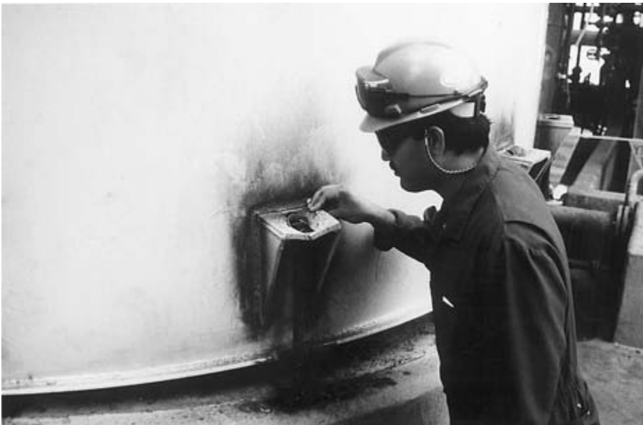
FIGURE 3-4 Tank bottom is bulged and anchor nuts are pulled through the anchor chairs.
