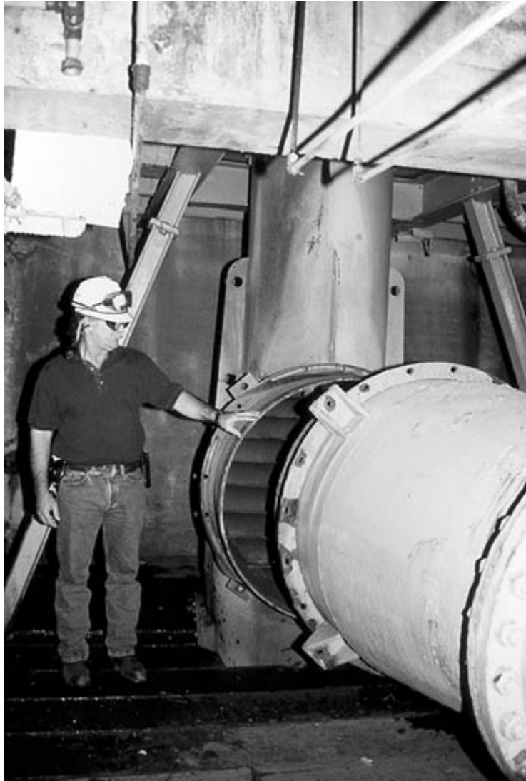
FIGURE 7-9 Photo of how the river water pump moved during the explosion.
