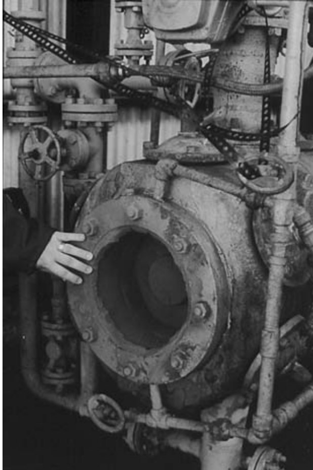
FIGURE 7-2 Close-up of ruptured water jacket on compressor.
