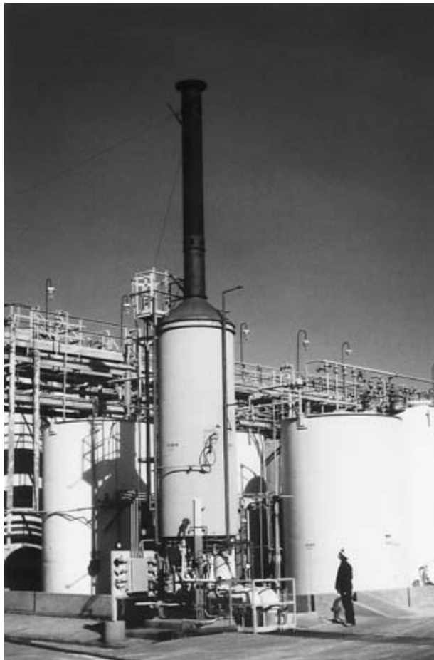
FIGURE 6-4 The rejuvenated and relocated gas-fired heater.
