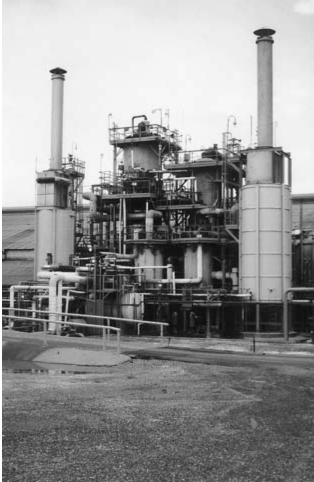
FIGURE 6-5 Well-maintained unit is troubled by a leak.
