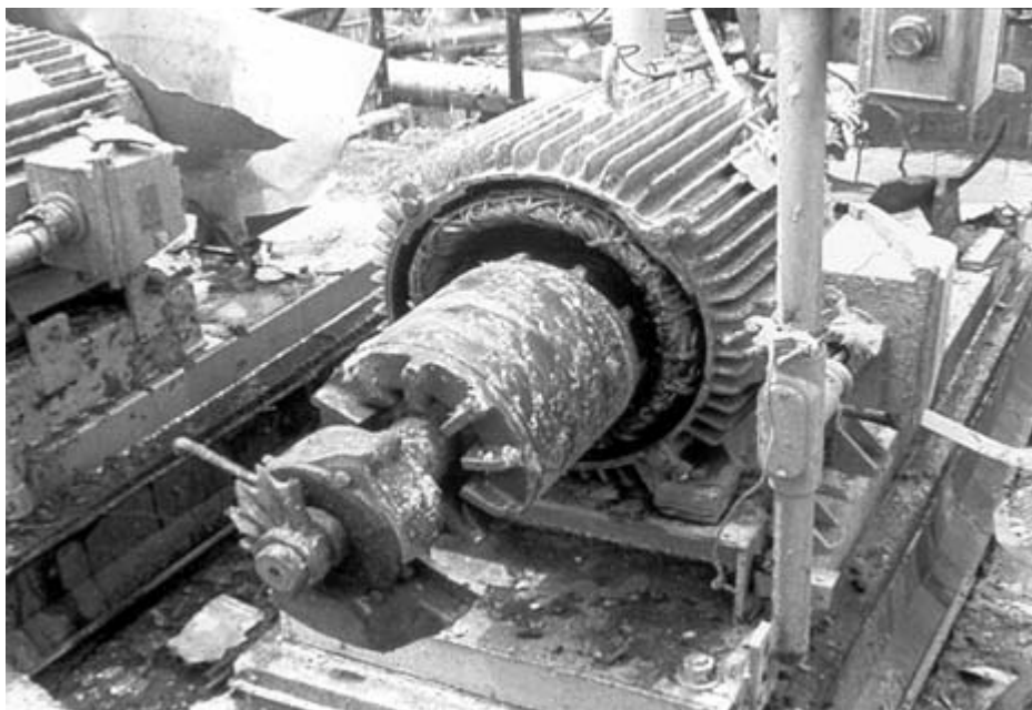
FIGURE 7-16 Explosion forces rotor out of condensate pump motor. Courtesy of Eastman Chemical Company.
