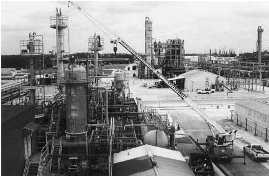
FIGURE 10-19 A crane is lifting a recently tested and reconditioned safety relief valve to reinstall on a reactor.
