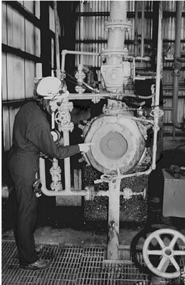
FIGURE 7-1 Reciprocating compressor with ruptured water jacket.
