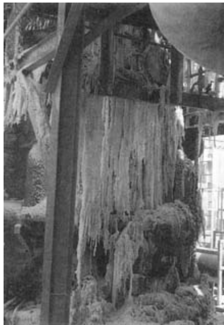
FIGURE 6-7 Icicles are formed from leaking caustic soda that dripped from an evaporator flange.
