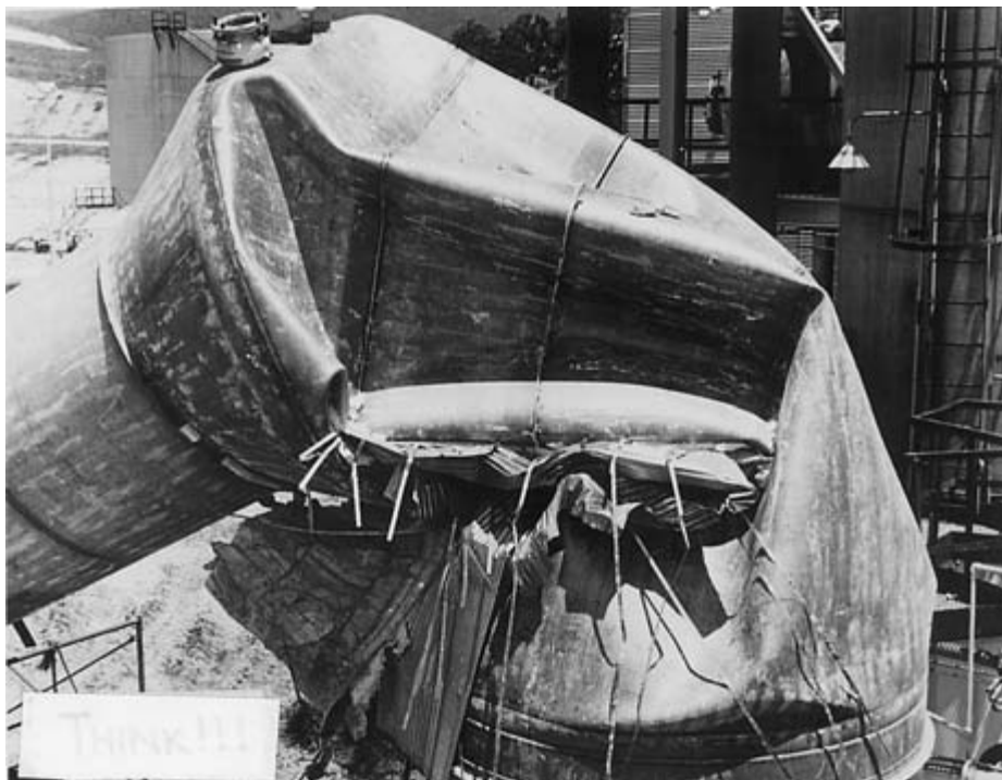
FIGURE 3-7 A close-up of a collapsed stripper column. Courtesy of Guido DeJesus.
