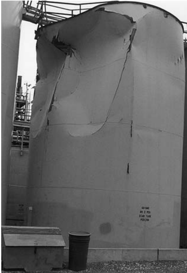
FIGURE 2-13 A 12-ft.-diameter tank ruined after vent system is improved.
