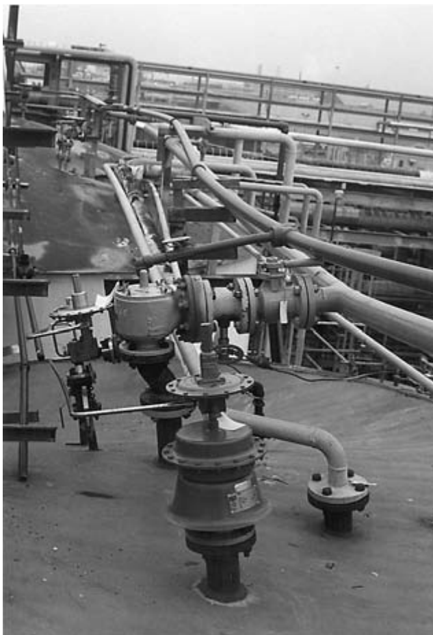
FIGURE 2-15 New but visually confusing piping system—after the incident.
