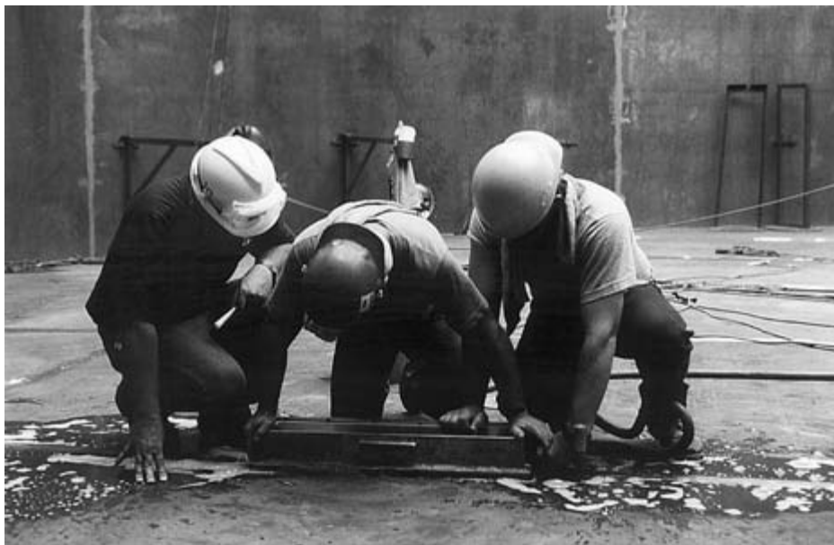
FIGURE 10–13 Inspectors using a vacuum box and soapy water to check for leaks in welds on the floor of low-pressure tanks.
