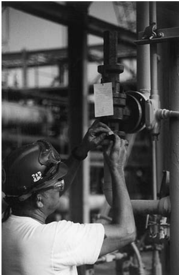
FIGURE 10–17 A mechanic is removing an SRV from a unit. The mechanic records the condition of the inlet and outlet piping components on the tag before the valve is sent for testing.
