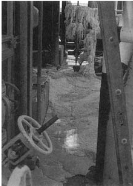
FIGURE 6-6 Molten caustic soda leaks from above due to an improper gasket.
