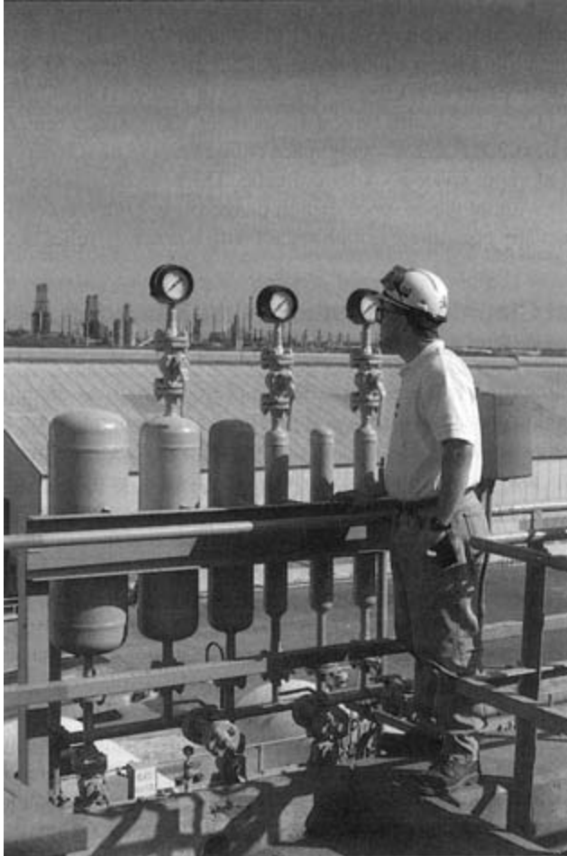
FIGURE 4-5 An engineer observes the pressure gauges on chlorine expansion bottles.
