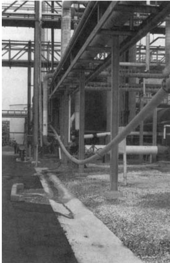
FIGURE 4-6 Pipe hangers corrode and pipe drops to the ground.
