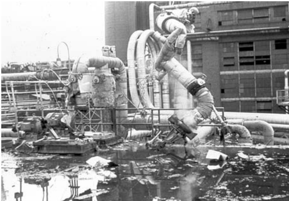
FIGURE 7-15 Heavily damaged condensate pump installation. Courtesy of Eastman Chemical Company.
