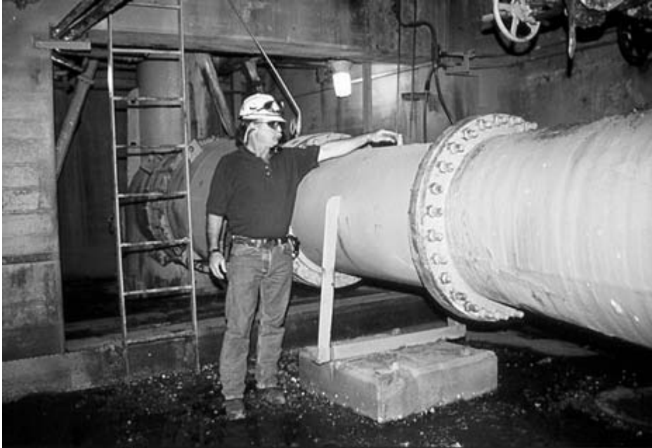
FIGURE 7-7 Photo of the adjacent river water pump system.
