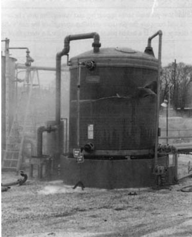
FIGURE 2-8 Acid tank just after failure.
