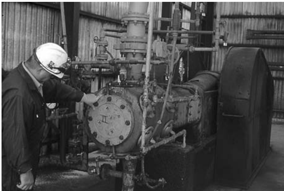
FIGURE 7-3 Rebuilt reciprocating compressor.
