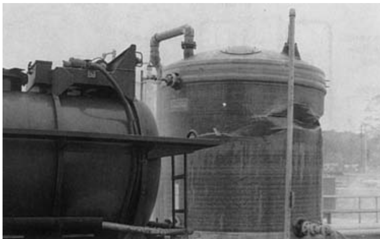
FIGURE 2–7 Tank truck parked next to damaged acid tank.
