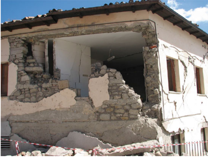
Fig. 20.36 Partial overturning of a multi story wall, Accumoli 2016
