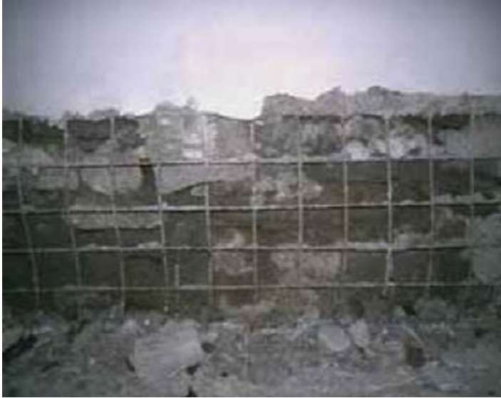
Fig. 20.73 Degradation of the reinforced plaster due to a lack of connection of the welded grid to the wall
