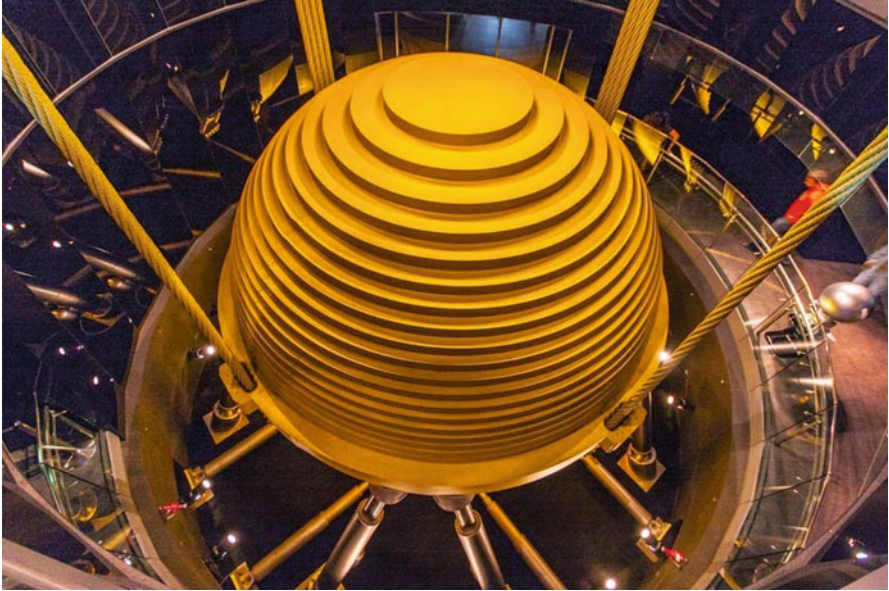
Fig. 18.12 TMD inside at Taipei 101
