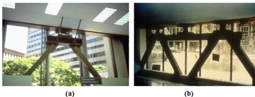
Fig. 17.7 ADAS system implementation in Wells Fargo building, San Francisco (a) Izazaga building, Mexico City (b)
