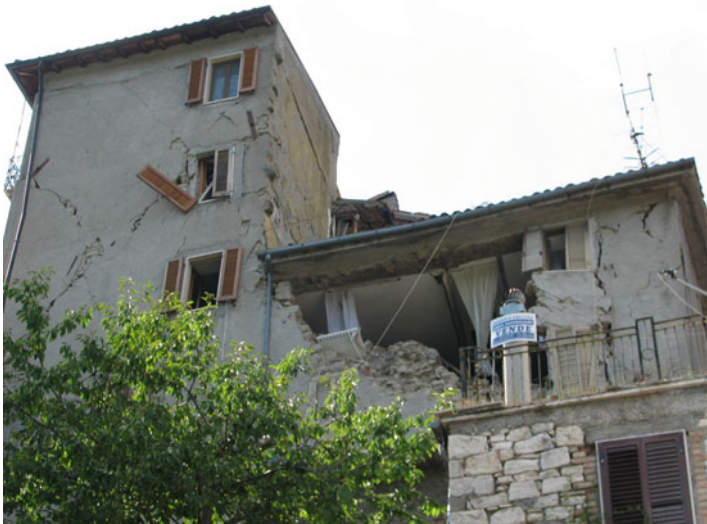
Fig. 20.20 Damages due to discontinuity along the height, Arquata 2016
