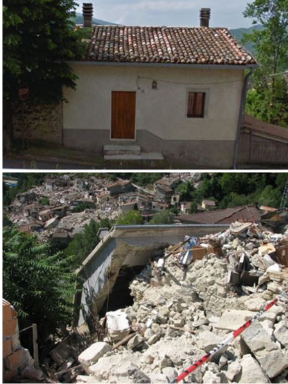
Fig. 20.47 Overturning of the reinforced concrete roof. Pescara del Tronto, 2016
