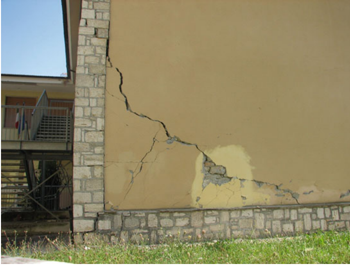
Fig. 20.24 Settlement of the foundations, Arquata 2016
