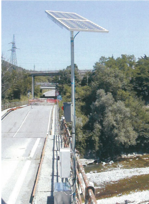
Fig. 8.4 DMS system equipped with automatic acoustic/visual alerting devices
