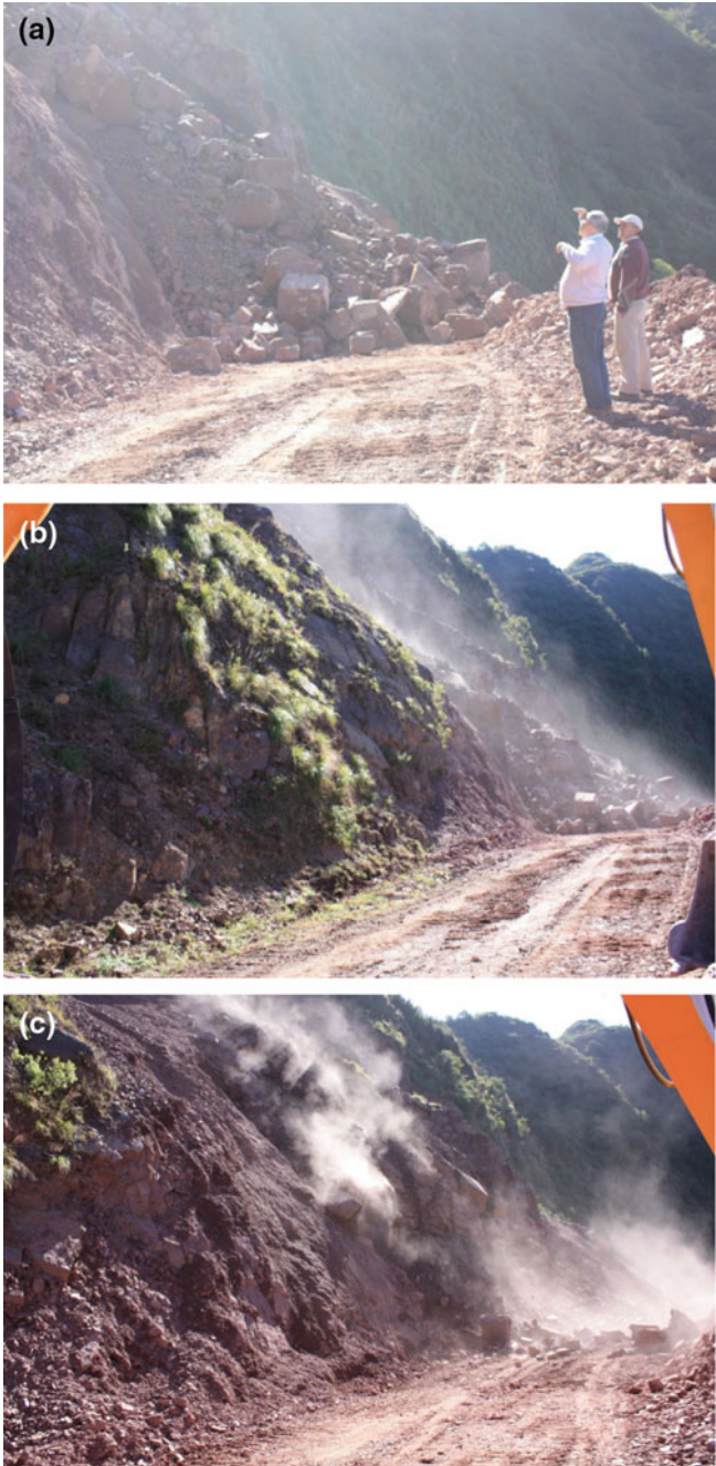
Fig. 6.22 a–c Explosion of marly rock, very fractured, happened live on 9.5.2010 after three days of persistent rainfall on the southern slope near Quebrata del Toro—ancient road—Yuyui Province, Argentinian Pre-Andes
