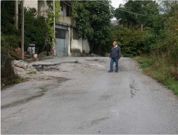
Fig. 5.46 Effects of the landslide to the upslope
