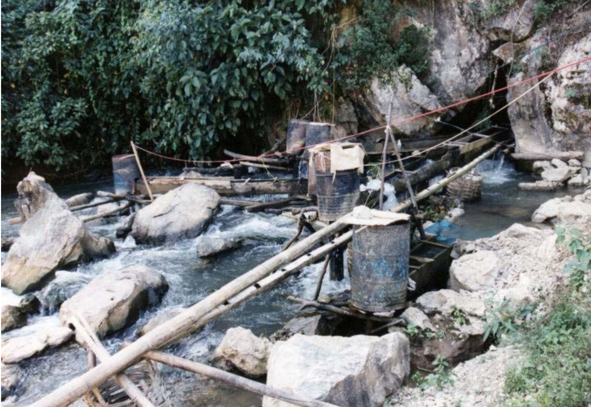
A micro-hydro facility in Vietnam.
