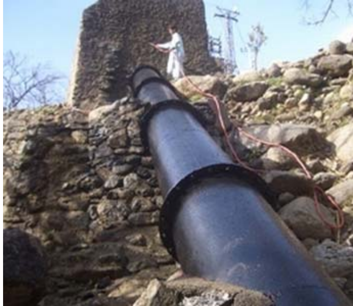
A penstock pipe used in an Afghanistan micro-hydro project
