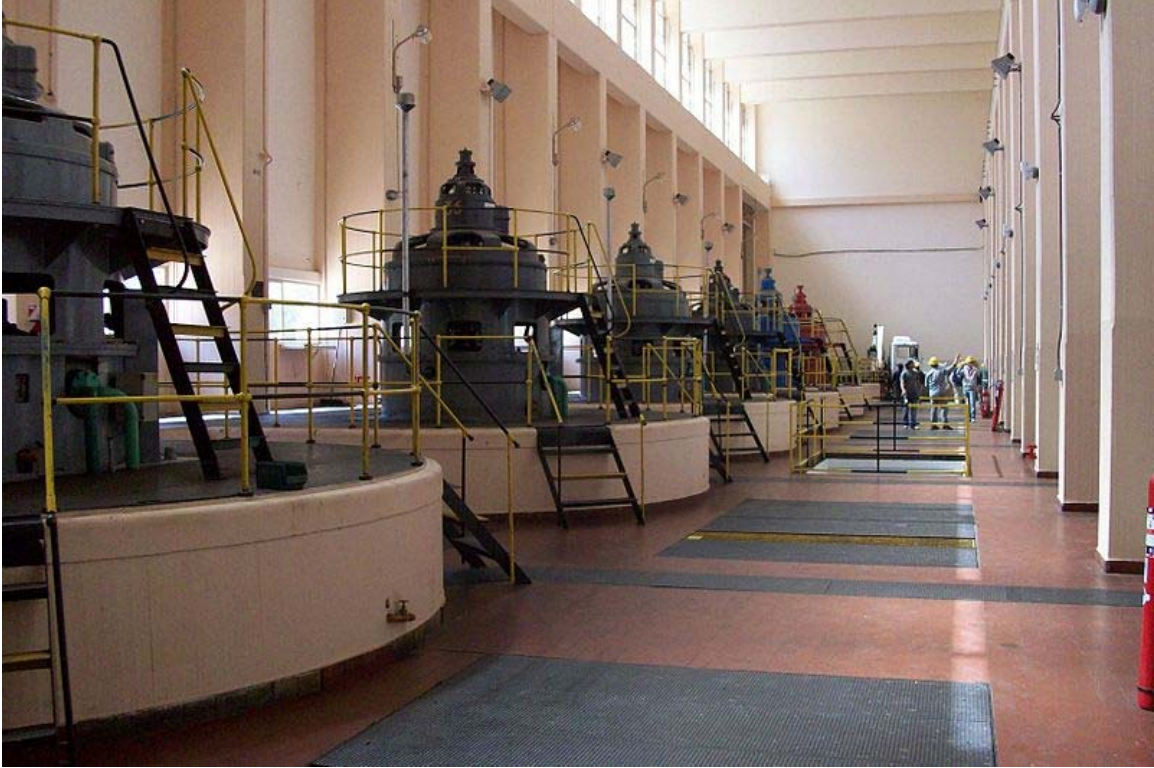
Turbine row at Los Nihules Power Station in Mendoza, Argentina
