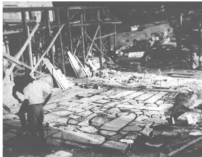
2 Construction of pavement in front of St. Dimitrios church. (Photograph Agni Pikionis)
