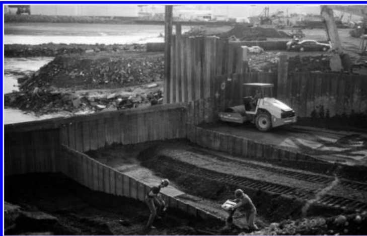
FIGURE 9.A9 Open Cell being backfilled. (Courtesy of John W. Pickering, PE, MBA, President, PND Engineers, Inc.)
