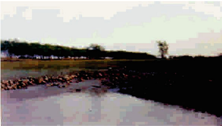
Fig. 17.11 Bank condition after 20 years
