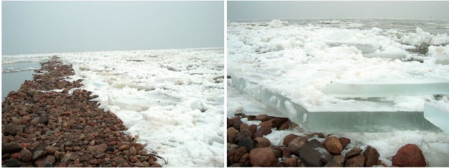
Fig. 2 Ice rubble in the Vistula Outlet acting on the west jetty (January 2003)
