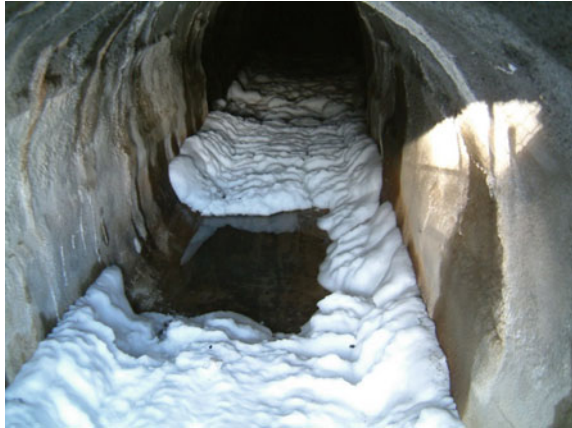
Fig. 10 Accumulated ice on the floor of a water-diversion tunnel after the tunnel was drained
