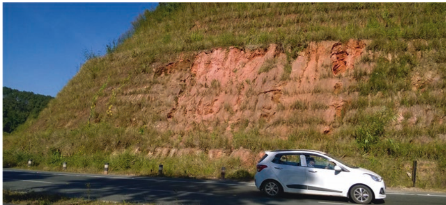
Fig. 19.7 Stabilization of cut slope as of July 2015 by vetiver grass along Guwahati–Shillong National Highway, Meghalaya State, India
