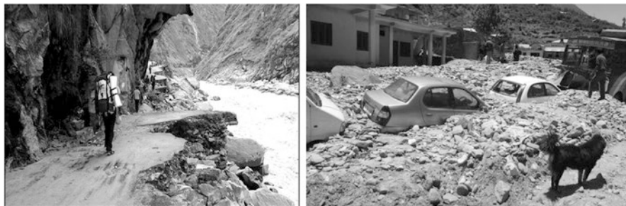
Fig. 9.4 View of road disruption in June 2013 due to bank erosion in the proximity of Tawaghat, Pithoragarh ( left ), and debris slide in Dharali, Uttarkashi ( right )
