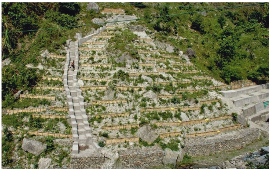
Fig. 19.2 Application of bamboo check dams for retaining water and concrete drain as one of the indigenous slope stabilization measures at Kalimpong, West Bengal (Photo: http://savethehills.blogspot.in/ )
