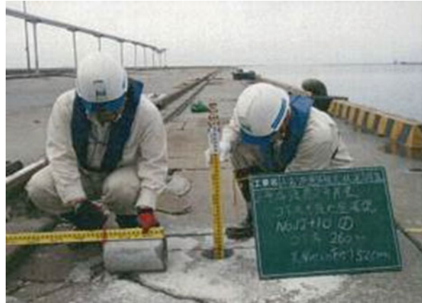
Fig. 13.8 Damage state photograph of the quay wall at No.3-wharf in Onahama port
