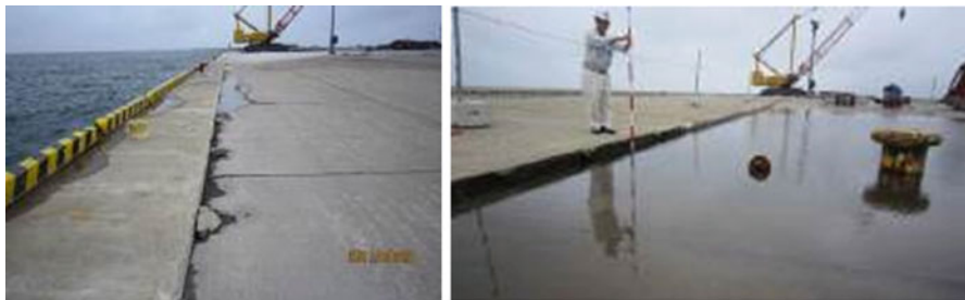
Fig. 13.6 Damage state photographs of the quay wall at No.2-wharf in Soma port
