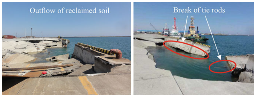
Fig. 13.3 Example of severely damaged quay walls due to combined disaster in Soma port, after Takahashi et al. (2011)
