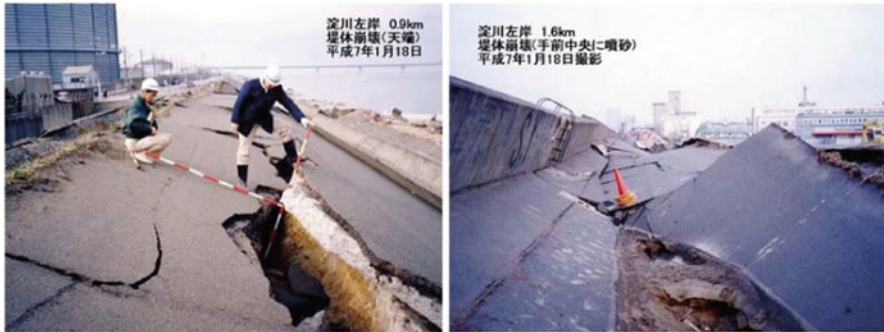
Fig. 8.20 Dyke suffered from the Hyogo-ken Nanbu Earthquake in 1995 (Website of Kinki Regional Development Bureau, /Yodogawa River Office http://www.yodogawa.kkr.mlit.go.jp/activity/maintenance/earthquake/ )
