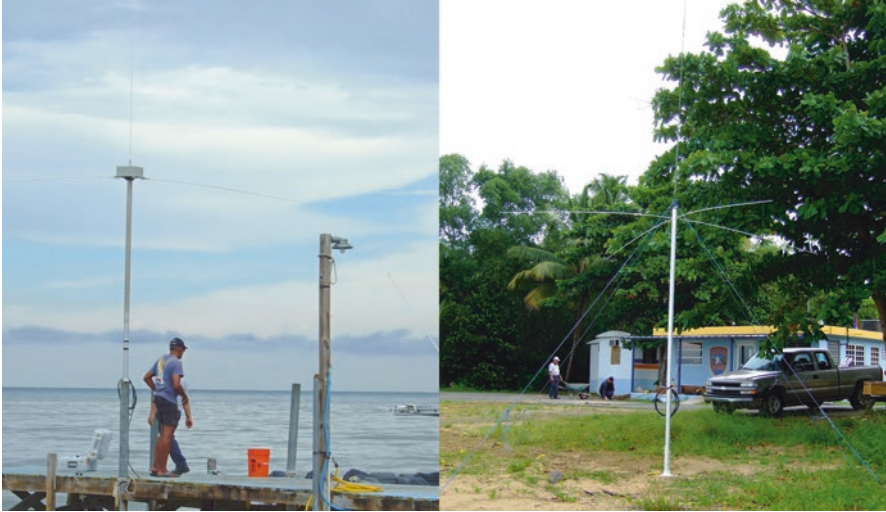
Fig. 2.4 Installing a high frequency surface current radar antenna emplacement on the west coast of Puerto Rico. Left: The receiving antenna mounted at the end of a dock. The housing at the top of the support mast holds orthogonal induction coils (see Fig. 2.5). Right: Transmit antenna mounted on the beach. Workers in the background are burying the Rx antenna cable run. Omnidirectional Tx and Rx antenna are mounted vertically and ground planes extend laterally
