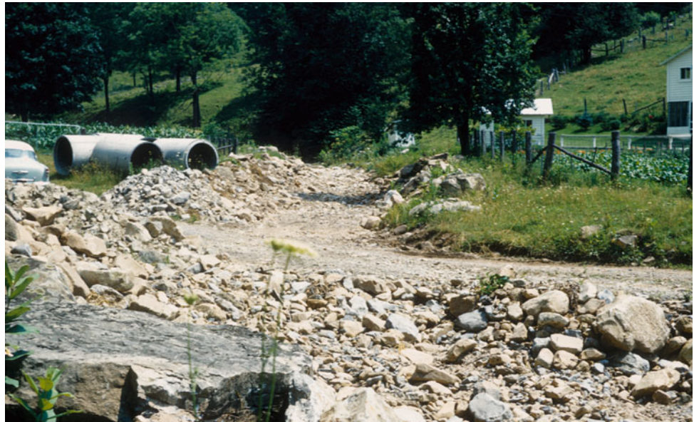
Fig. 6.3 Bed of dry Creek after storm flow has washed out the road. Note cobble and boulder fill in the stream bed. The bedload moves during extreme flood flow. Photo by W.B. White
