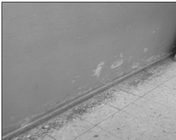
Figure 2. Wet areas in floors and walls.
