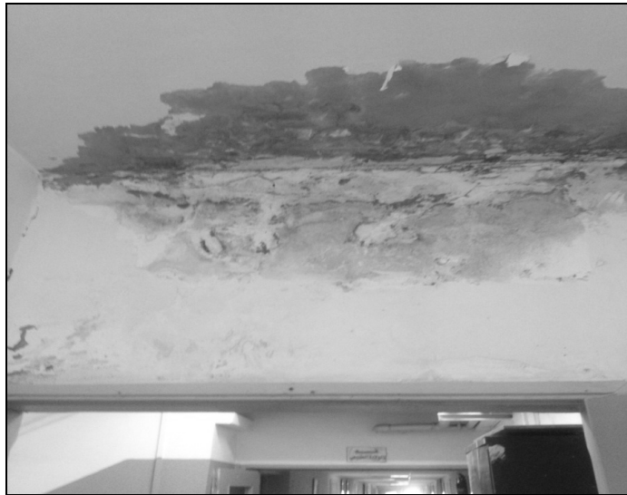
Figure 1. Wet areas in walls and ceilings.
