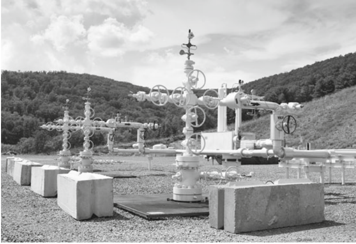
A shale gas well installation in Pennsylvania.
