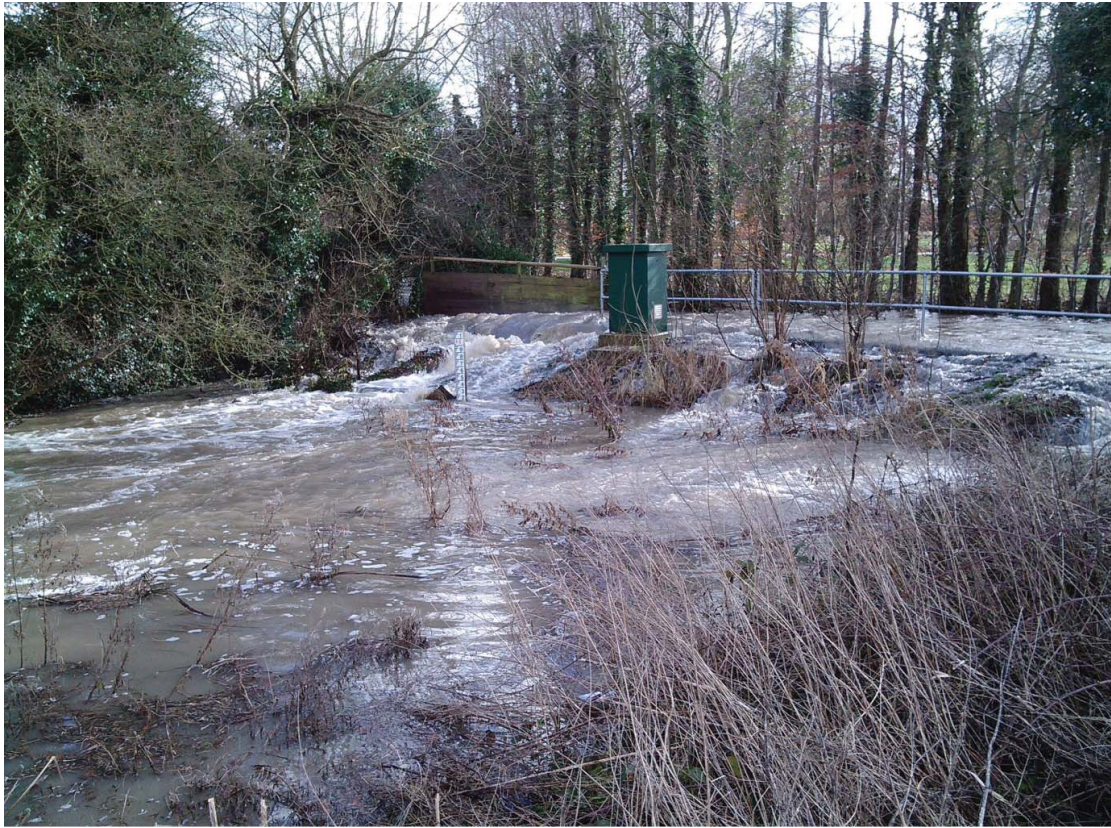
Fig. 3.2 A flooded gauging station. (Source: Reproduced with permission of Hydro-GIS Ltd.)
