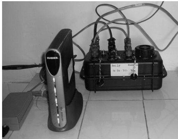
Fig. 2.4 VSAT communication indoor unit and DAS at field station
