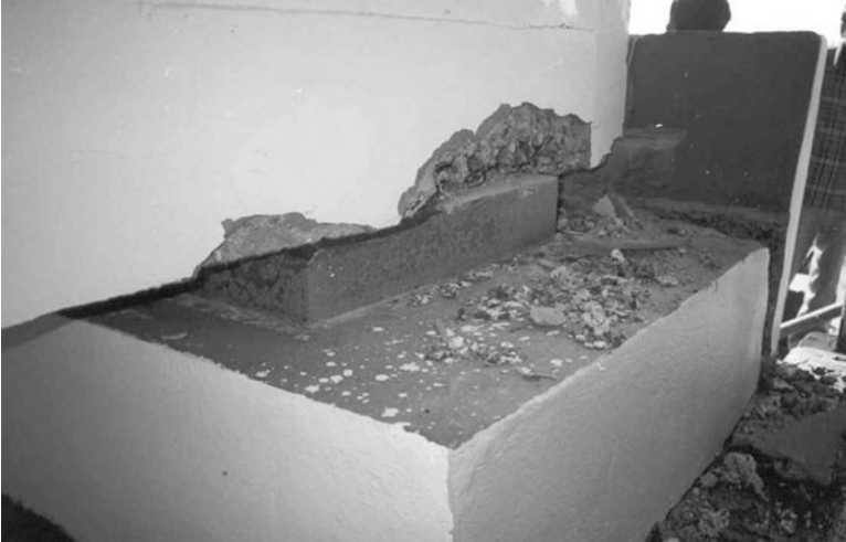
Fig. 10.3 Girder shifted in the longitudinal direction with loss of seating during shaking
