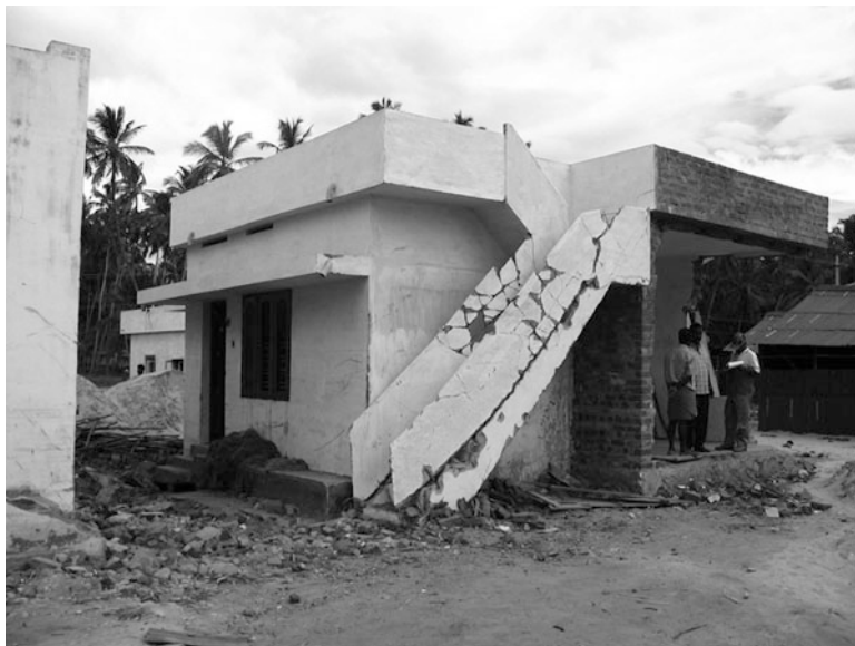
Photo 5.3 Damaged brick masonry building at Colachel
