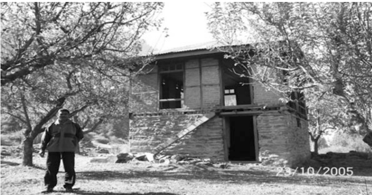
Fig. 14.2 Timber bands in a masonry building, Baramulla (Courtesy Mrs. Amita Sinvhal, Dept. of Earthquake Eng., IIT Roorkee)
