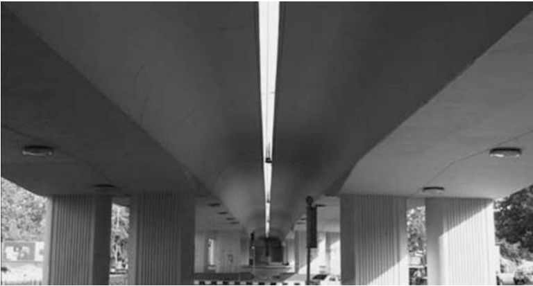
Fig. 10.7 Panchsheel Club Flyover, New Delhi piers and deck are monolithic
