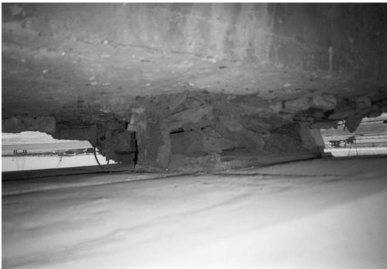
Fig. 10.2 Surajbari old bridge: Metallic bearings destroyed during earthquake
