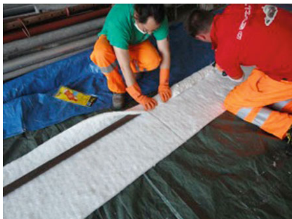
Fig. 3.13 Thermal insulation activity of the prop with insulating material consisting of alkaline earth silicate wool
