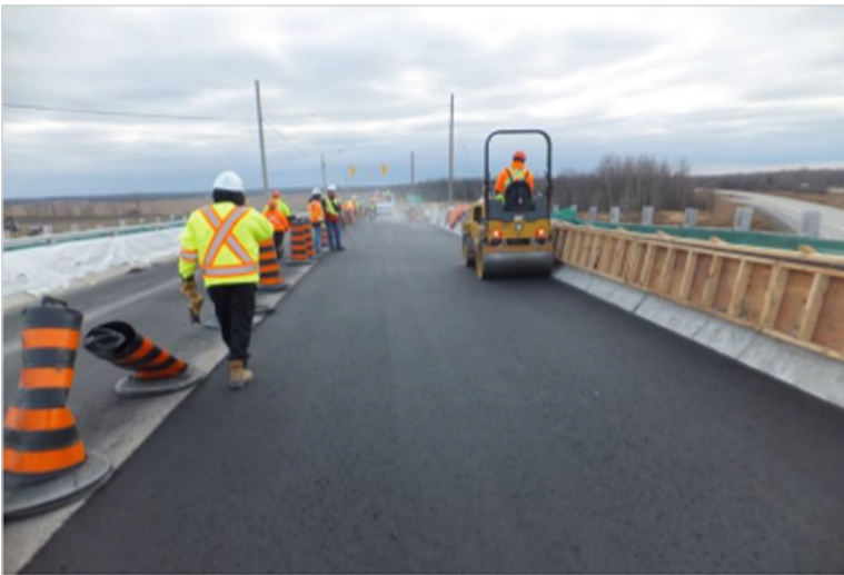
Fig. 5. Steel static roller compacts the edge of AMIR compacted lane, Highway- 34 Bridge
