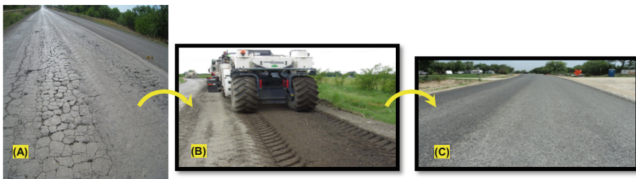
Fig. 1. (A) Deteriorated roadway (B) full depth reclamation (FDR) (C) opening the rehabilitated roadway to traffic in the same day
