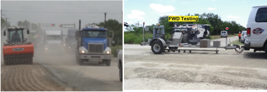
Fig. 6. Traffic condition during FDR construction and FWD testing on top of foamed asphalt treated base
