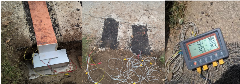
Fig. 10. Field installation and data collection
