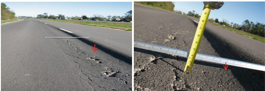
Fig. 3. Premature failure-occurred within one month of trafficking
