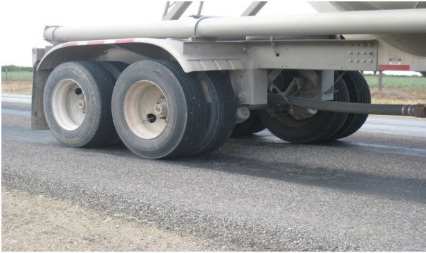
Fig. 4. A recent premature failure (deep rutting) due to insufficient early strength from FDR layer
