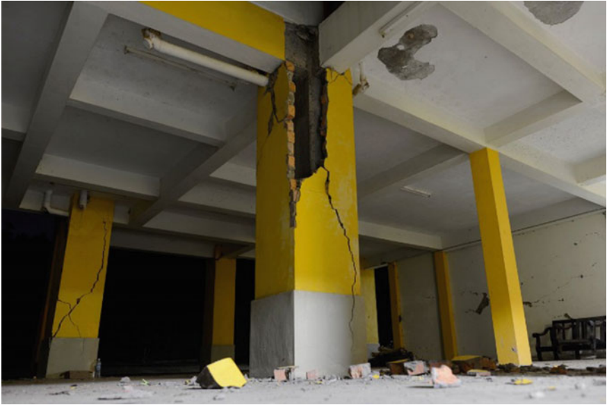
Fig. 1. The damaged column under seismic loading [4]
