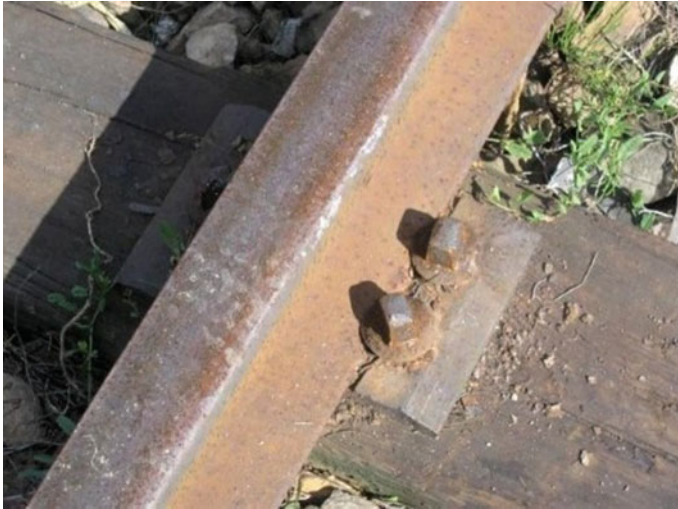
Fig. 8.1 An example of a direct, rigid fastening of rails to the wooden sleepers ( http://www.transportszynowy.pl/kolprzytw1bezp.jpg )
