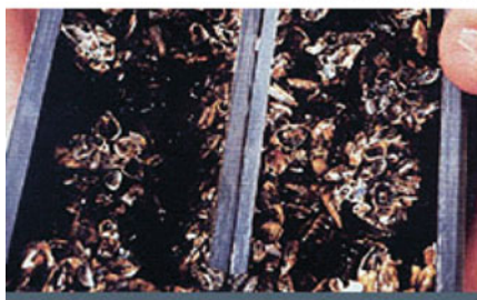
Zebra mussels in power plant pipe
