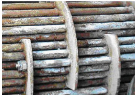
Heat exchanger tubing with crystallization
