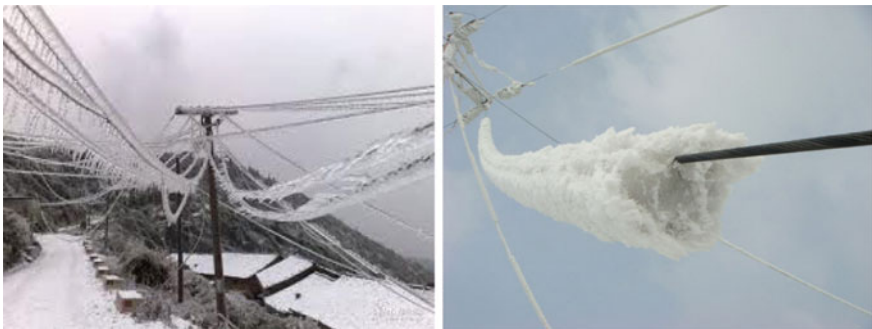
Fig. 15.4 Ice formed on the power cables in snow blasting in January 2008 Southern China (from public domain)
