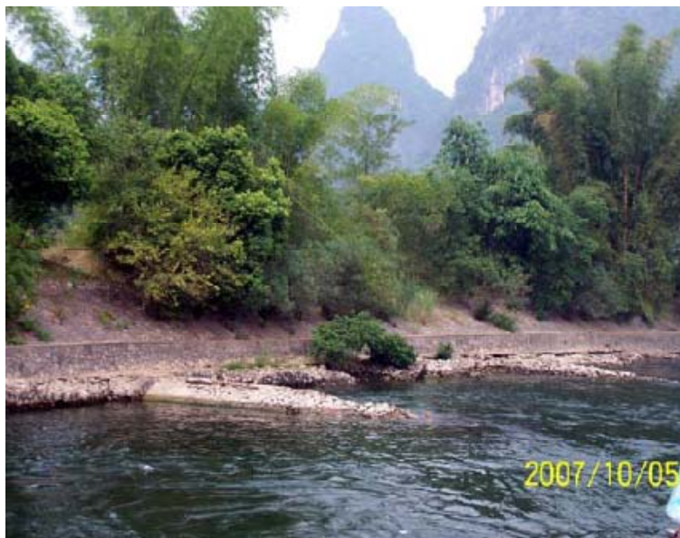
Figure 48. Spur dikes on the Lijiang River in south China used to promote the formation of low velocity habitats.
