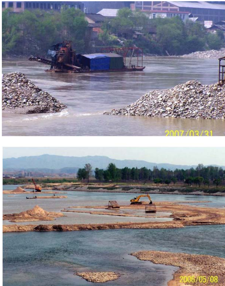
Figure 28. (a) Gold placer mining in the Bailong River, a tributary of the Jialing River in Sichuan; (b) Gravel mining for building materials from the Qingjiang River, a tributary of the Yangtze River.
