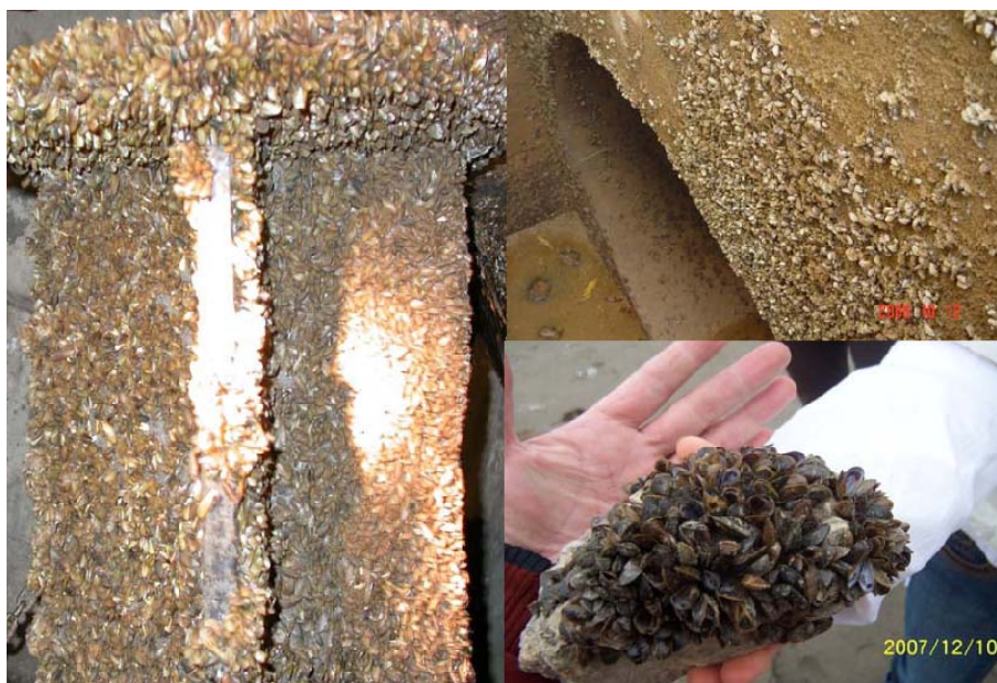
Figure 37. Colonization of golden mussel on concrete walls in a water transfer tunnel and attachment of golden mussel on a concrete fragment with high density.
