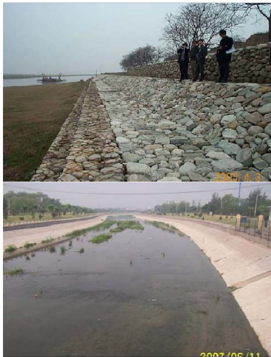
Figure 23. (a) Hardened banks of the Weihe River; (b) Concrete banks and bed of an urban stream in Beijing.
