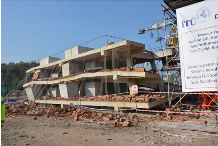
Fig. 22.9 Collapsed reference building
