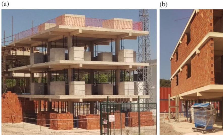
Fig. 22.5 Views of test buildings, concrete weight blocks and infill walls during construction process (Tore et al. 2017)
