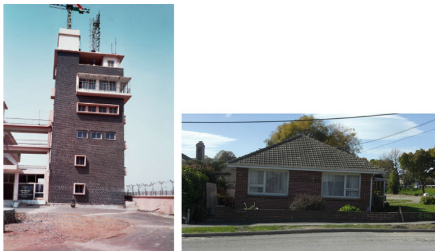
Fig. 16.10 Settlement and rotation of a tall structure and a residential structure due to soil liquefaction
