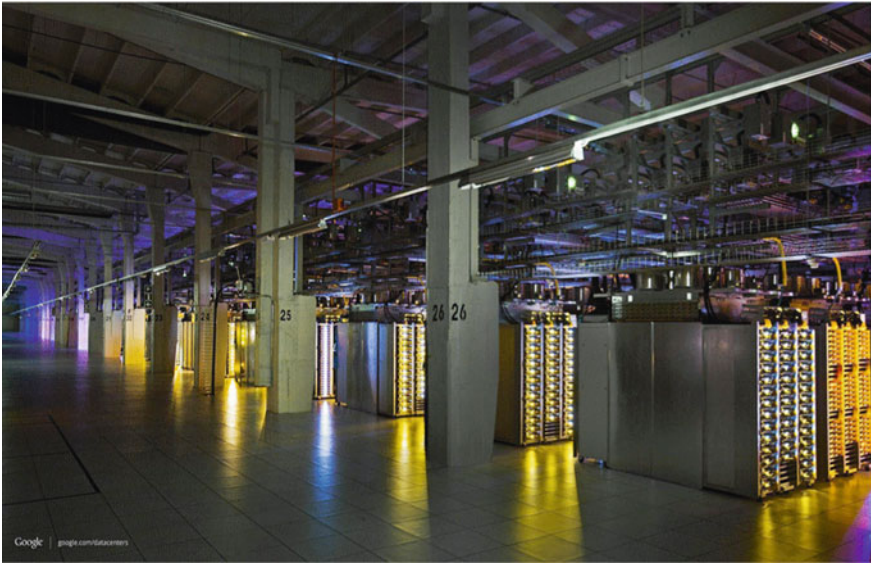
Fig. 17.1 Inside a Google datacenter, showing rows of racks, each rack housing tens of servers. Optical interconnections from the server racks can be seen above them, going to cable trays which house the fibers ( http://www.google.com/about/datacenters/ )
