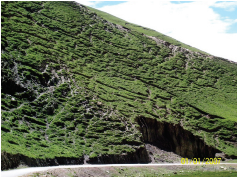
Figure 2.34 Local-scale cracks or cavitations due to swelling and shrinking along the Qinghai-Tibet Highway.
