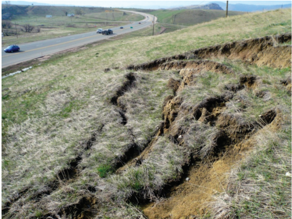
Figure 2.33 Tensile cracking developed near the top of a hillslope in Jefferson County, Colorado.
