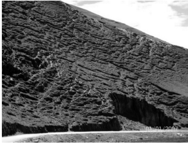
Figure 2.34 Local-scale cracks or cavitations due to swelling and shrinking along the Qinghai-Tibet Highway. See also color plate section.
