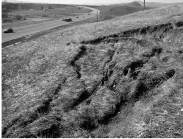
Figure 2.33 Tensile cracking developed near the top of a hillslope in Jefferson County, Colorado. See also color plate section.
