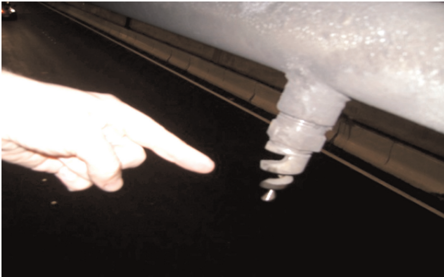
Figure 4.2 A spiral nozzle located in the area where the tunnel fires occurred
