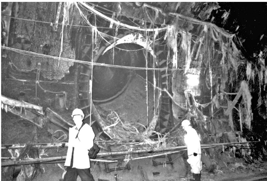
Figure 2.1 Fire damage to the tunnel around a piston relief duct. (Photograph courtesy of the author)
