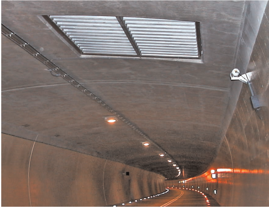
Figure 9.13 View of single point extraction damper in tunnel roadway (Katschberg Tunnel, Austria) (Reproduced by permission of Peter Sturm of the Technische Universität Graz)
