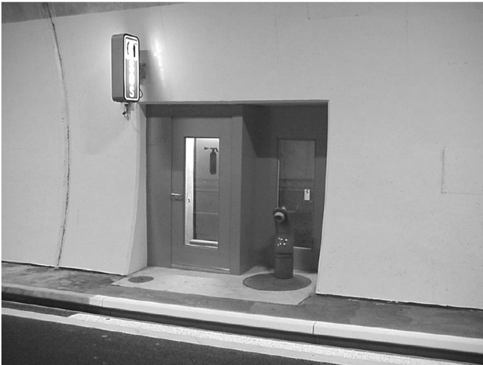
Figure 21.5 Emergency station with fire extinguisher, emergency phone and hydrant
