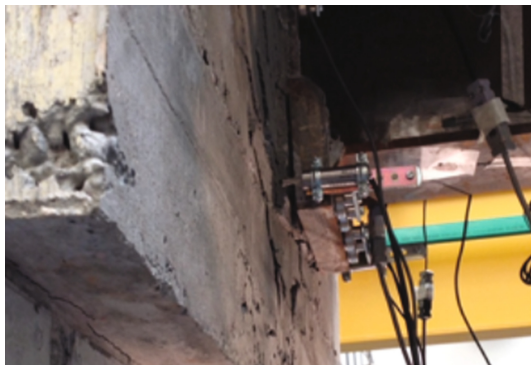
Fig. 13. Detachment of the steel girder end plate
