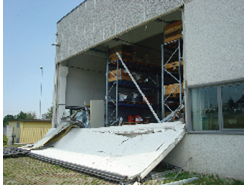
Fig. 1. Emilia 2012 – panel collapse
