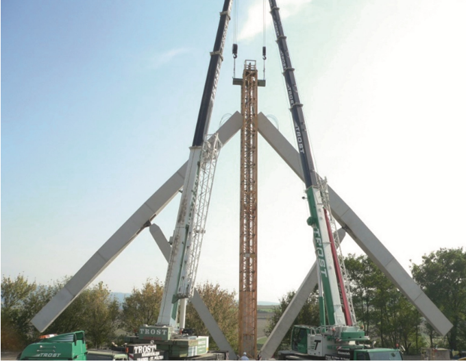
Fig. 14. Lowering of the top points of the bridge girders with the aid of mobile cranes
