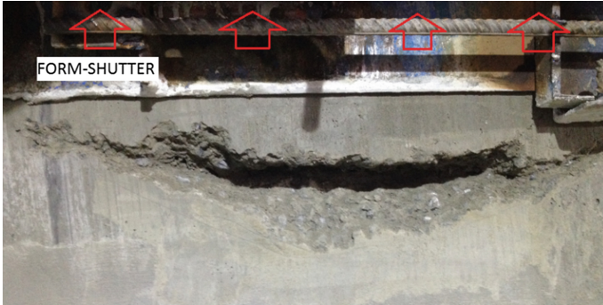
Fig. 14. Moke-up: superficial concrete tear
