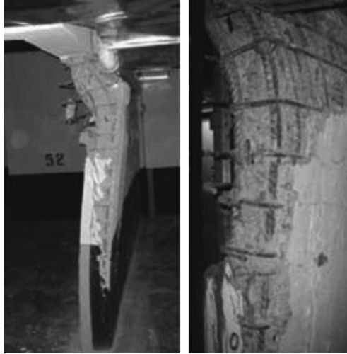
Fig. 1. Out-of-plane buckling of walls after 2010 Chile earthquake (Wallace 2012)
