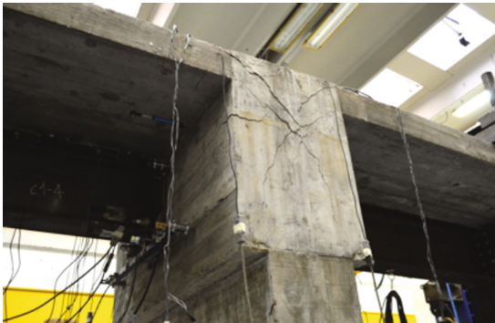
Fig. 12. Crack pattern in the CCB
