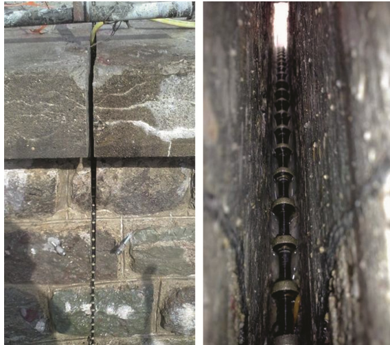
Fig. 12. The slot cutting from downstream face. On the left, the kerb of the crest; on the right, the wire in the middle of the cutting.
