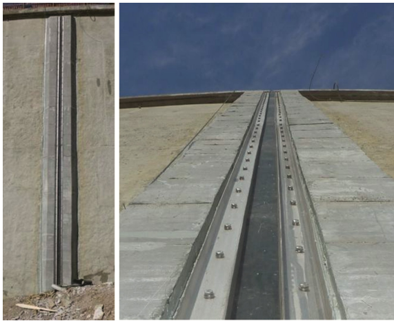
Fig. 13. The new joints. On the right, the detail of the superficial part of the complex removable sealing device.
