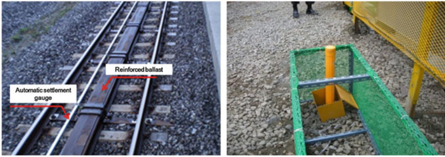
(a) Automatic settlement instrument (b) Inclinometer
