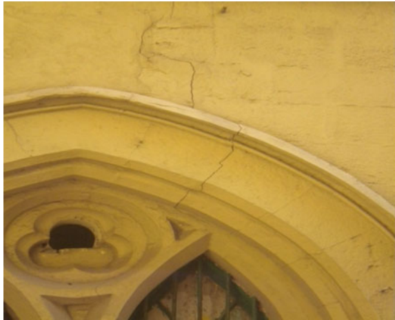
Fig. 1 A view of cracks in wall (outer view of N–W wall)
