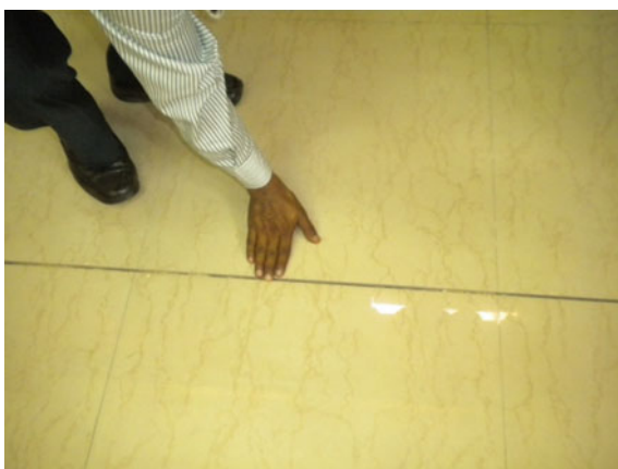
Fig. 4 Differential settlement in floor
