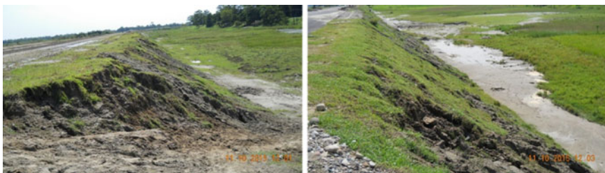
Fig. 9 Embankment slopes in October 2016, eroded by run-off during rainfall
