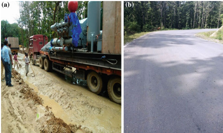
Fig. 8 a Heavy vehicles plying over the granular base over the geocells. b The repaired stretch in July 2017
