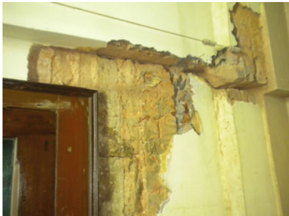
Fig. 2 Damage seen on the wall
