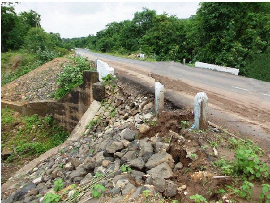
Fig. 3 Typical stone pitching damage
