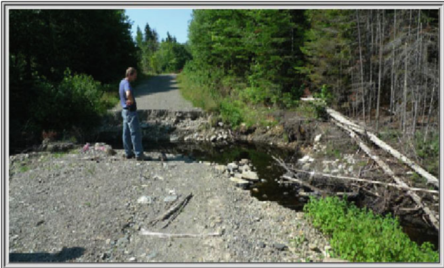
Fig. 1 Road section washed away by flooding
