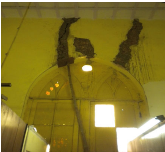
Fig. 3 Distinct cracks seen on wall (N–W) side
