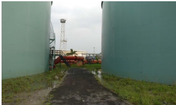
Plate 2 Photograph showing accumulation of water around the tanks and subsidence of the sand pad foundation below the ground
