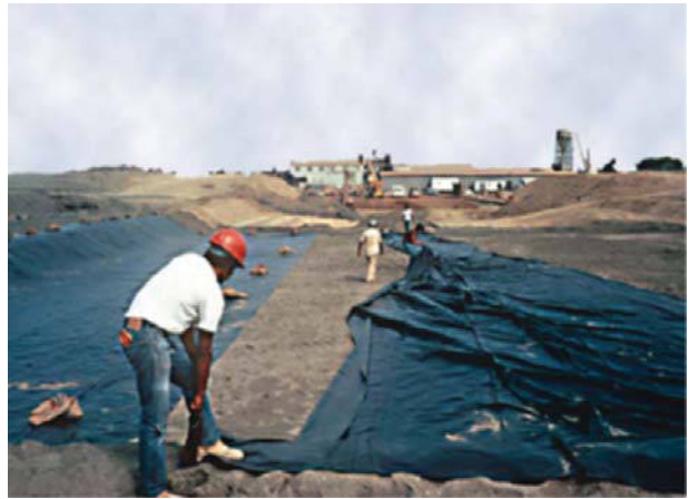
Figure 24.22 Installing a geomembrane in a bottom liner. (Courtesy of Layfield Environmental Systems, Layfield Group Limited, 11120 Silversmith Place, Richmond, British Columbia, Canada V7A 5E4.)
