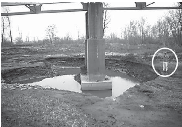
Figure 23.16 Scour hole around bridge pier.
