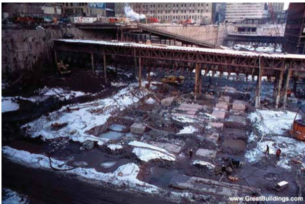
Figure 5.10 Photo of the foundation for the World Trade Center. (Courtesy of the Port Authority of New York and New Jersey.)
