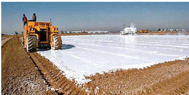
After applying lime slurry to prepared soil, the machine is run in reverse to ensure thorough mixing to the specified depth.
