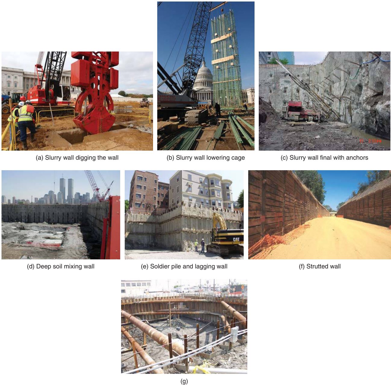
Figure 21.38 Various anchored and strutted wall techniques. (a, b, c, d: Courtesy of Nicholson Construction; e, f, g: Courtesy of Schnabel Foundation Company.)
