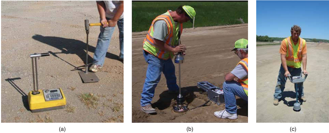
Figure 20.7 Compaction control tests in the field: (a) Nuclear gage. (b) Lightweight deflectometer. (c) BCD. (a: Photo by Lindsey D. Fields, Envirotech Engineering & Consulting, Inc. b: Courtesy of Minnesota Department of Transportation.)
