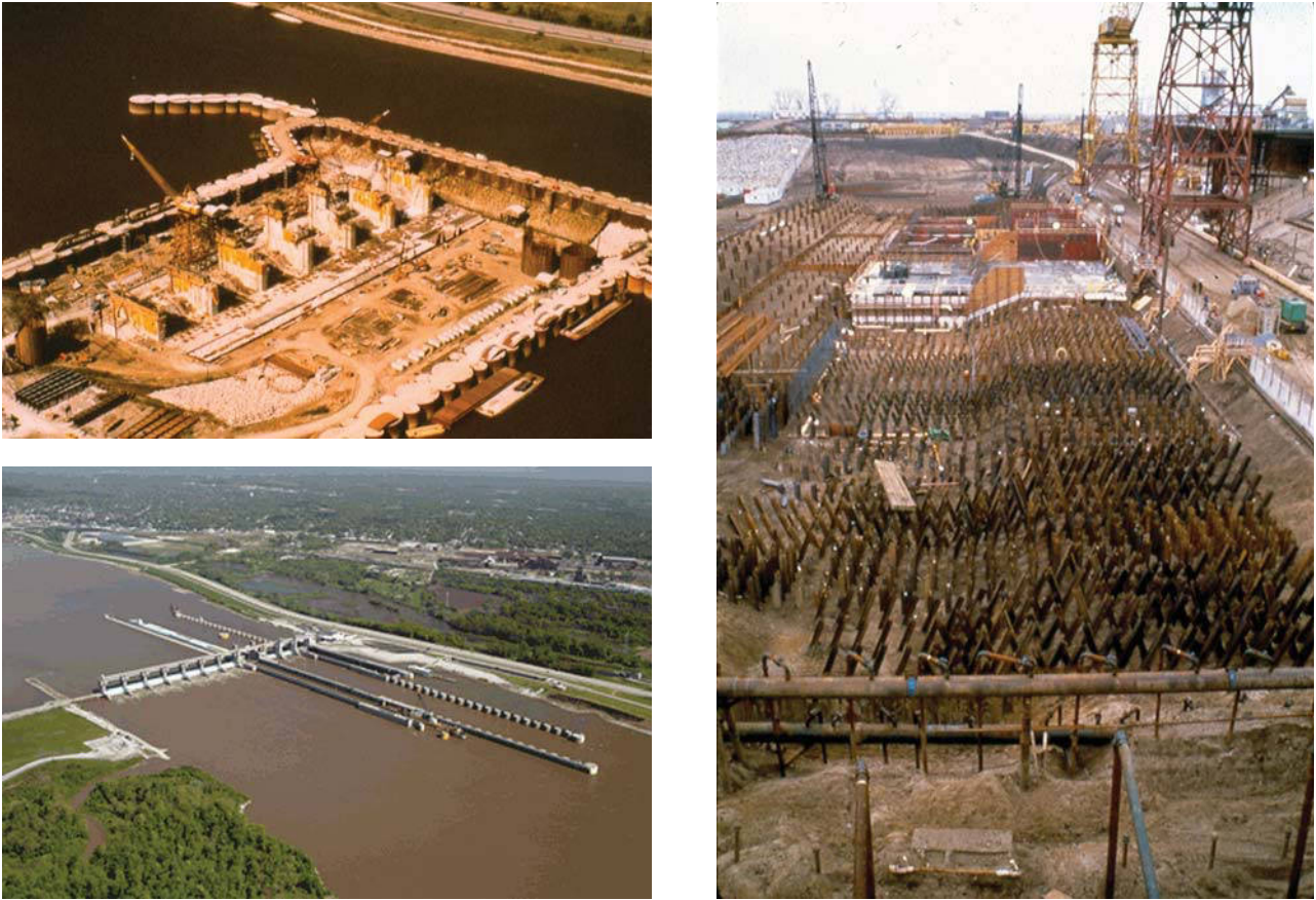
Figure 1.5 Lock and Dam 26 on the Mississippi River in 1990. (a: Courtesy of United States Army Corps of Engineers, b: Courtesy of Thomas F. Wolff, St. Louis District Corps of Engineers, 1981. c: Courtesy of Missouri Department of Transportation.)
