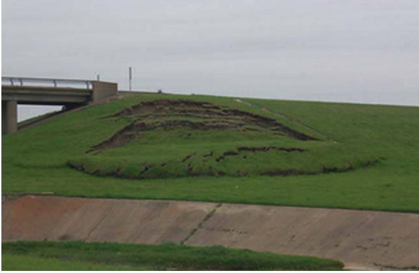
Figure 19.30 Shallow slide in a compacted embankment. (Courtesy of Professor Charles Aubeny, Texas A&M University.)
