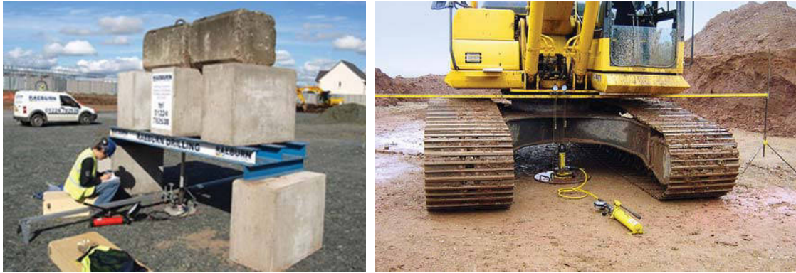
Figure 7.25 Plate load tests. (a: Photo by David Wilkins. Courtesy of Raeburn Drilling and Geotechnical (Northern) Limited; www.raeburndrillingnorthern.com . b: Courtesy of GEMTECH Limited, Fredericton, New Brunswick.)
